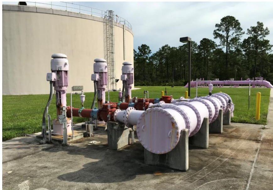
Exhibit 4 Existing Phase IV E-B PAR High Service Pump Station
