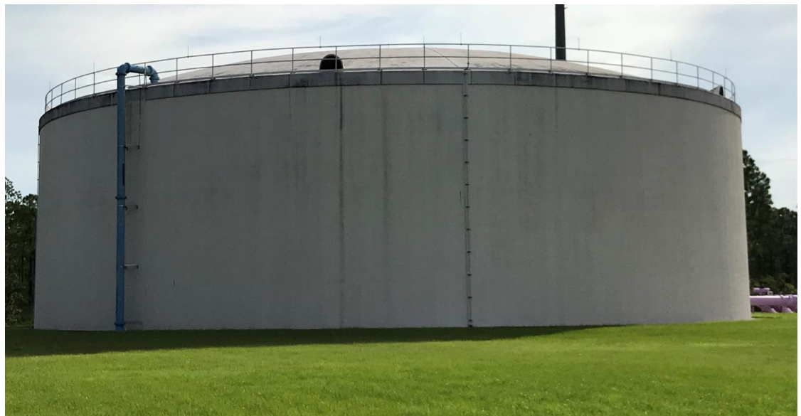
Exhibit 6 Existing Phase IV-B Ground Storage Tank with ASR Fill Piping
