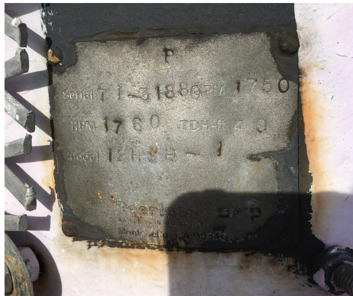
Exhibit 3 Existing Phase I/II Effluent Pump Nameplate
