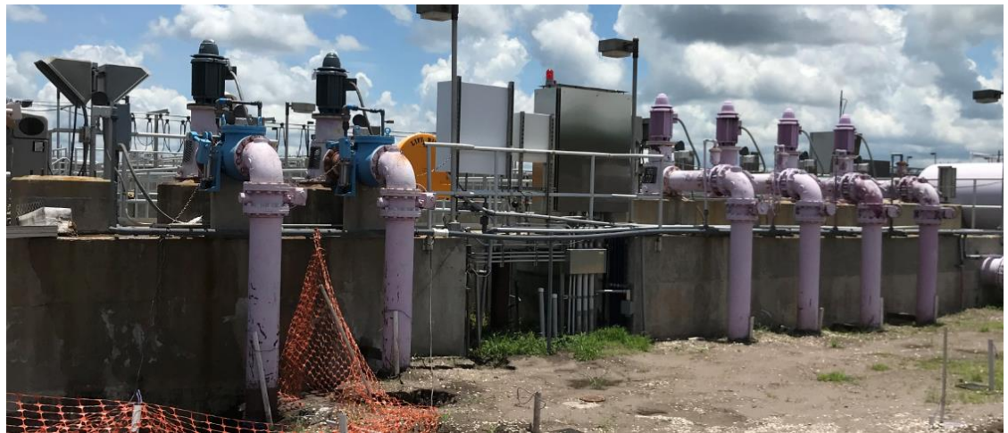
Exhibit 1 Existing Phase I/II Effluent Pump Station
