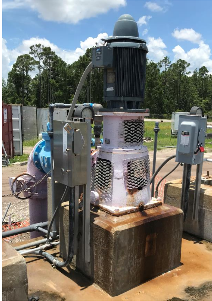
Exhibit 2 Existing Phase I Effluent Pump
