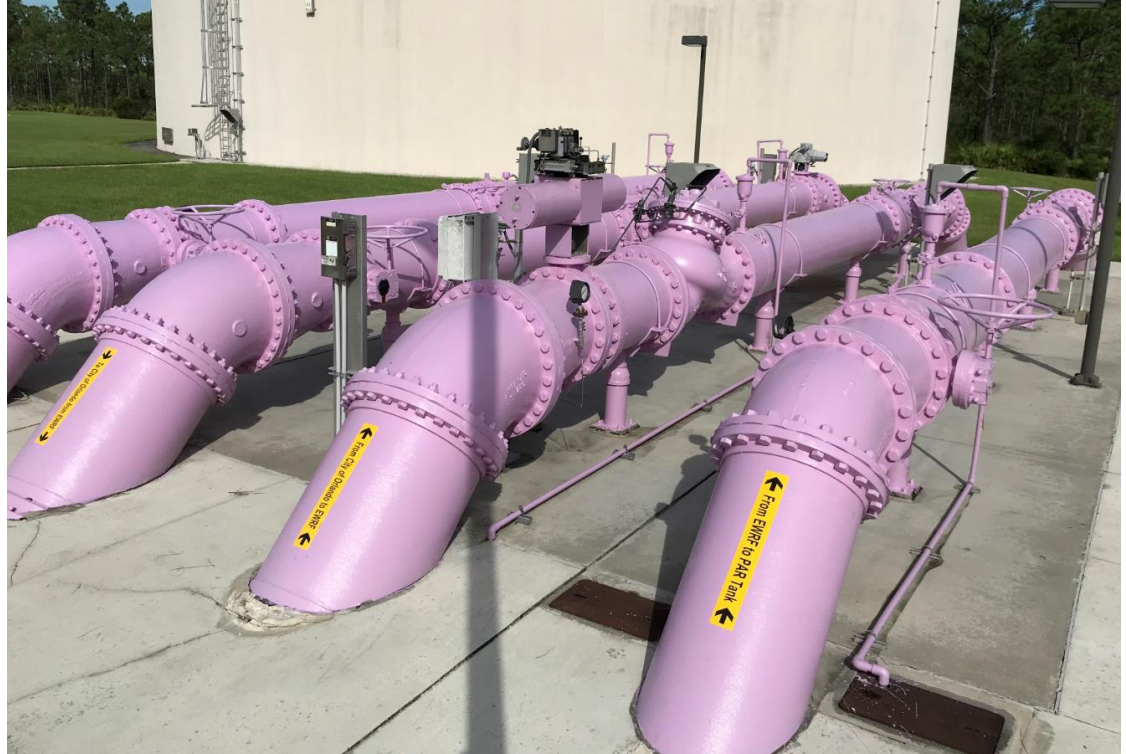
Exhibit 5 Existing Phase IV-B Meter Station
