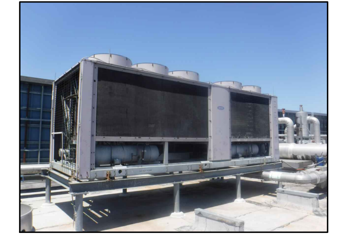
EXISTING CHILLER CH-2 TO BE REMOVED AND REPLACED
