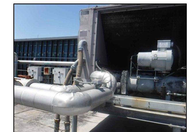
EXISTING CHILLED WATER SUPPLY AND RETURN PIPING TO BE REMOVED TO FIRST ELBOW
