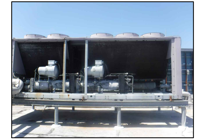
EXISTING CHILLER CH-1 TO BE REMOVED AND REPLACED
