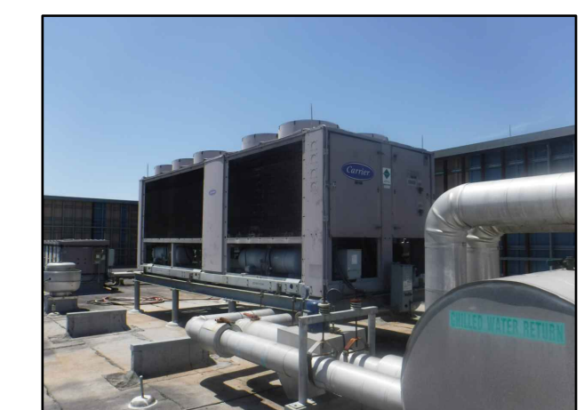
EXISTING CHILLED WATER SUPPLY AND RETURN PIPING TO BE REMOVED TO FIRST ELBOW
