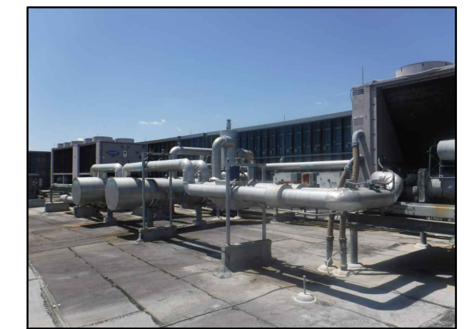
EXISTING CHILLED WATER SUPPLY AND RETURN PIPING, PRIMARY PUMPS AND ACCESSORIES TO REMAIN
