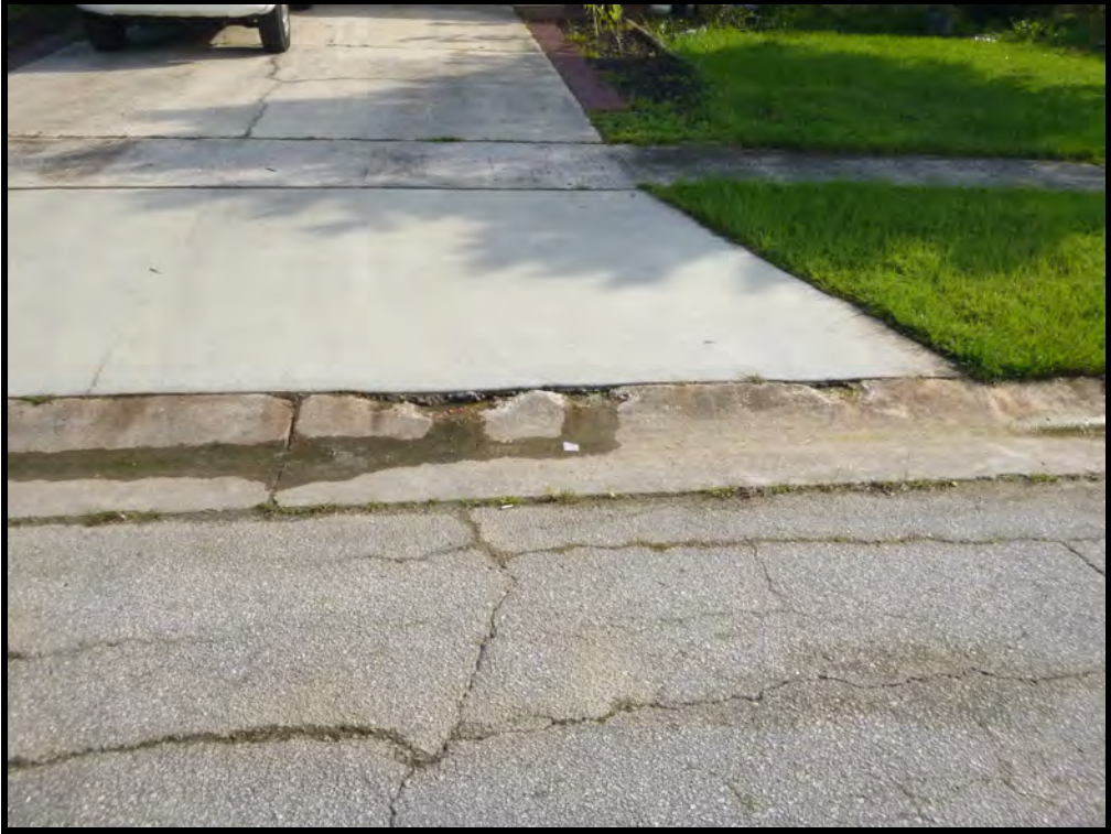
Photo #3. Seepage on Jepson Street
