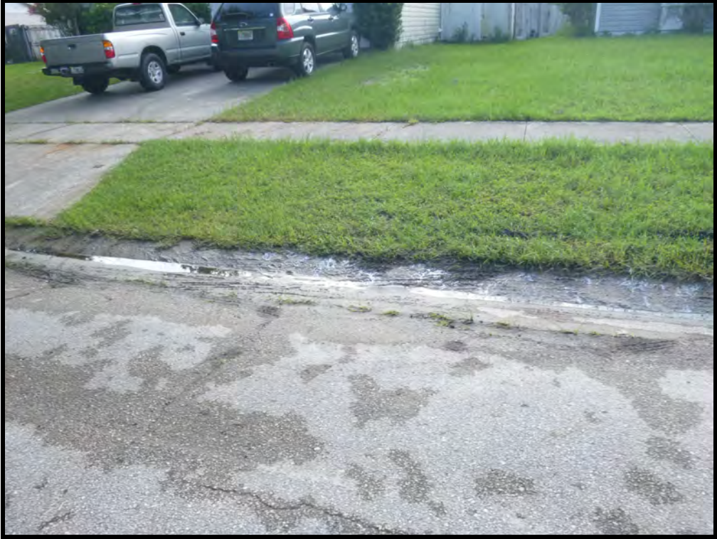
Photo #1. Seepage on Grayson Drive
