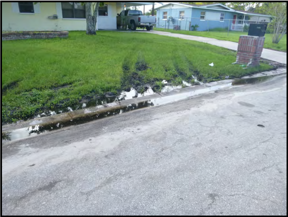
Photo #4. Seepage on Roberta Avenue
