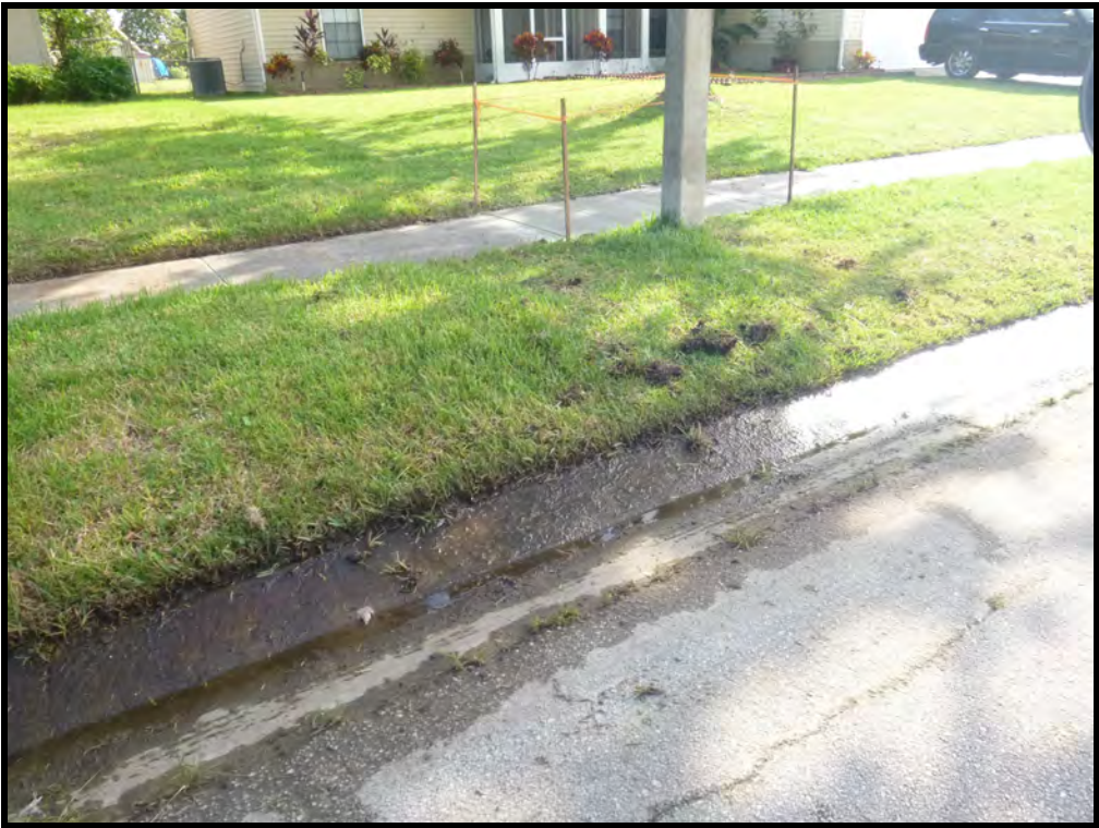
Photo #2. Seepage on Bridlewood Avenue
