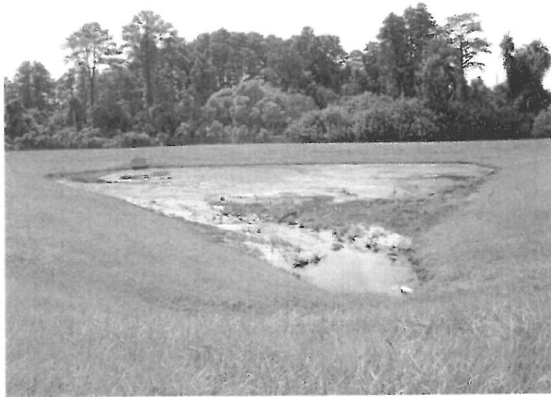
POND 7070 AND 7367- TURKEY LAKE ROAD, TRACT 922 LANDS DESCRIBED IN OFFICIAL RECORDS BOOK 4848, PAGE 1230 ORANGE COUNTY, FLORIDA
