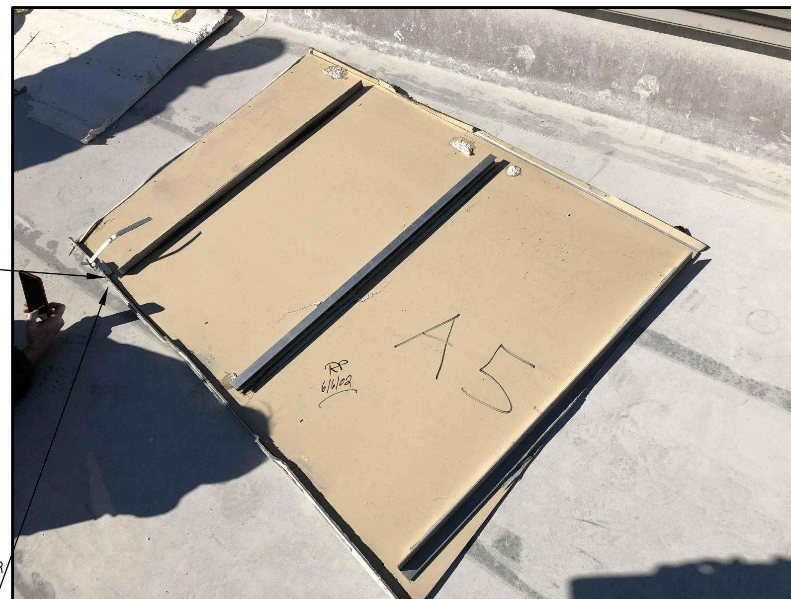
5 SOUTH BUILDING - EAST VAULT OR SOUTH B A01.01 VAULT STARTING PANEL BACKSIDE - STIFFENERS NTS
