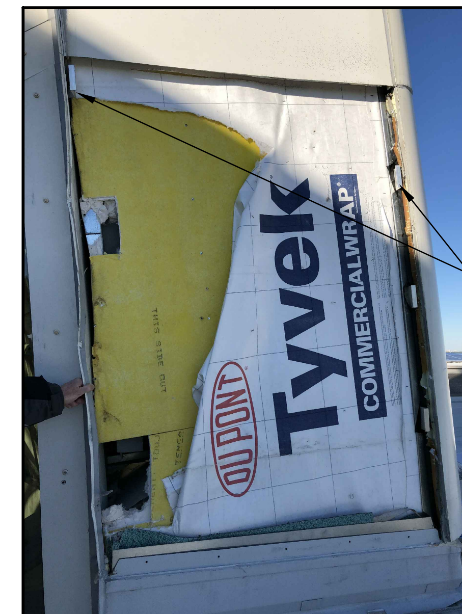
4 SOUTH BUILDING - EAST VAULT OR SOUTH B A01.01 VAULT STARTING PANEL VIEW LOOKING NORTH NTS
