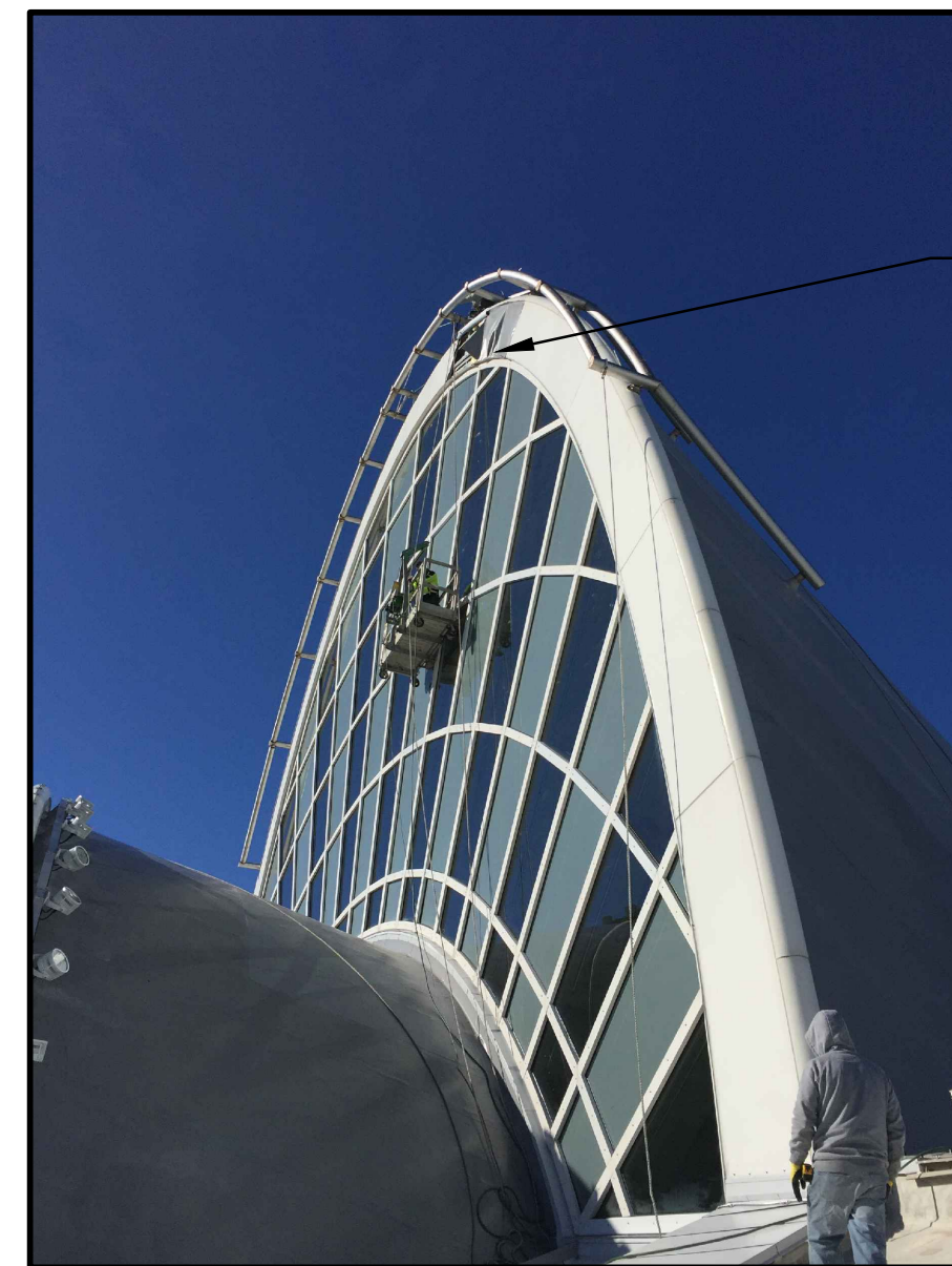
2 SOUTH BUILDING - EAST VAULT OR SOUTH B A01.01 VIEW LOOKING WEST NTS
