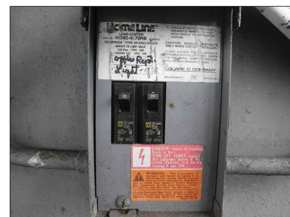
EXISTING PANEL "HHW3"
