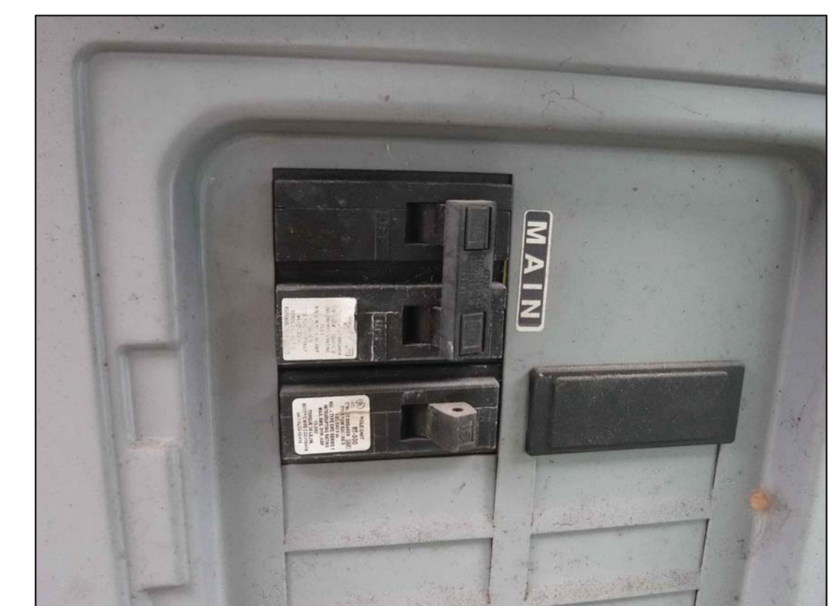
EXISTING PANEL "HHW2"
