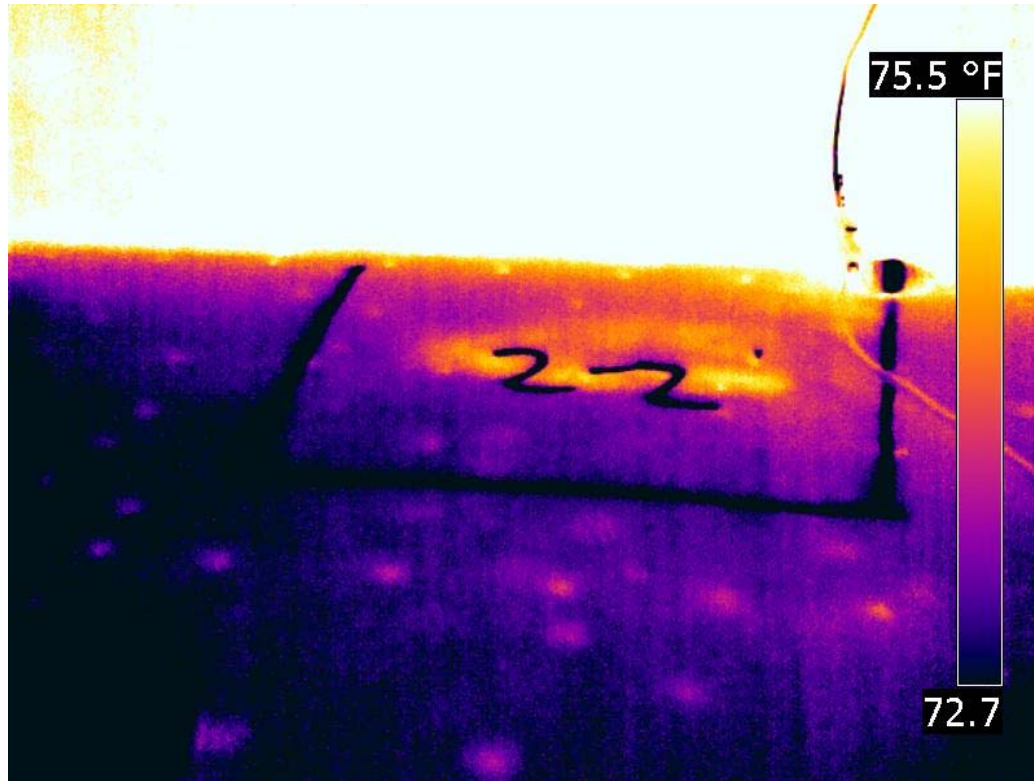
Infrared Image – light area shows location of trapped moisture
