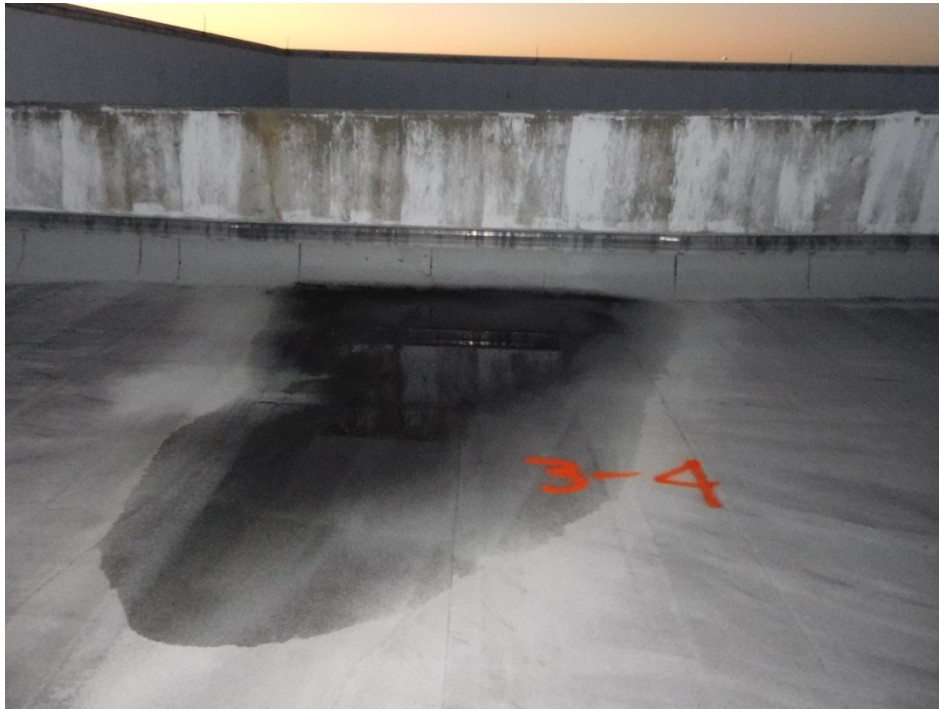
Visual Image of ponding water on roof
