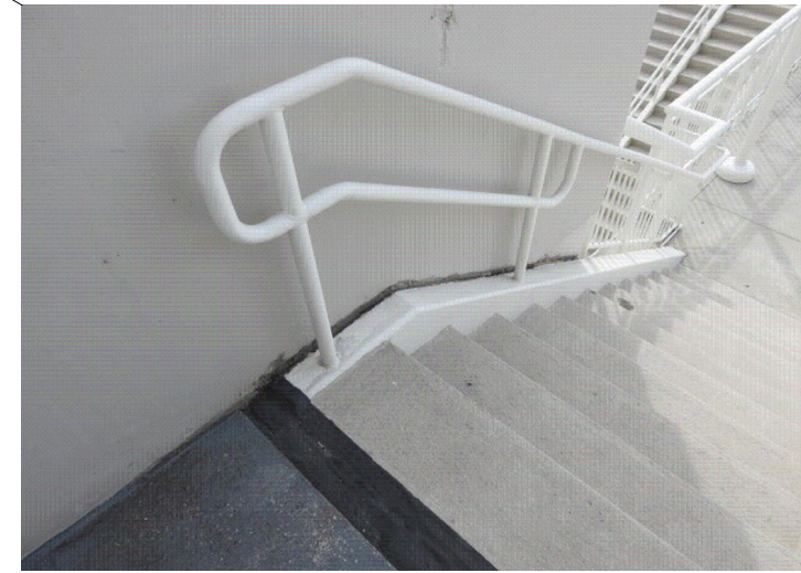
VIEW OF PARTIAL STAIR EXPANSION JOINT AND HANDRAIL EXPANSION JOINT COVER. THERE IS EVIDENT DETERIORATION OF THE JOINT AND COVER WHICH IS ALLOWING WATER INTRUSION TO THE LEVEL BELOW.
