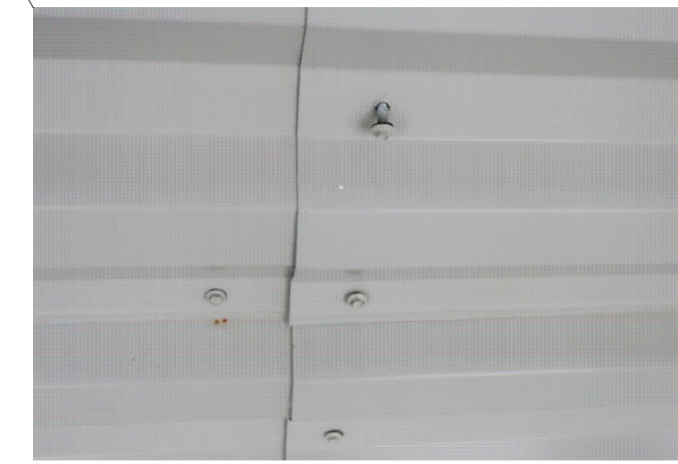
VIEW OF FASTENER BACKING OUT OF CORRUGATED STEEL. THIS OCCURS IN SEVERAL LOCATIONS AND WILL LIKELY ALLOW WATER INTRUSION AS WELL AS LIKELY CAUSE PANEL TO BECOME UNFASTENED FROM WALL. * THE REPAIR SCOPE SHALL BE AN "ADDITIVE BID ITEMS" ON THE WEST SIDE OF BUILDING ONLY *
