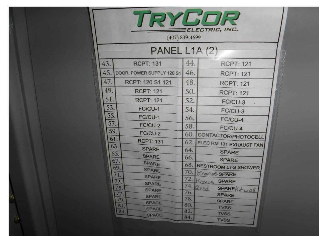
EXISTING 250 AMP PANEL WITH 250 AMP MAIN BREAKER ESTIMATED EXISTING CONNECTED LOAD ON TWO SECTION PANEL L1A(1)(2) IS 52.4KVA OR 146 AMPS. ESTIMATED ADDITIONAL CONNECTED LOAD FROM THIS SCOPE OF WORK IS 17.8KVA OR 49 AMPS FOR A NEW CONNECTED LOAD OF 195 AMPS.
