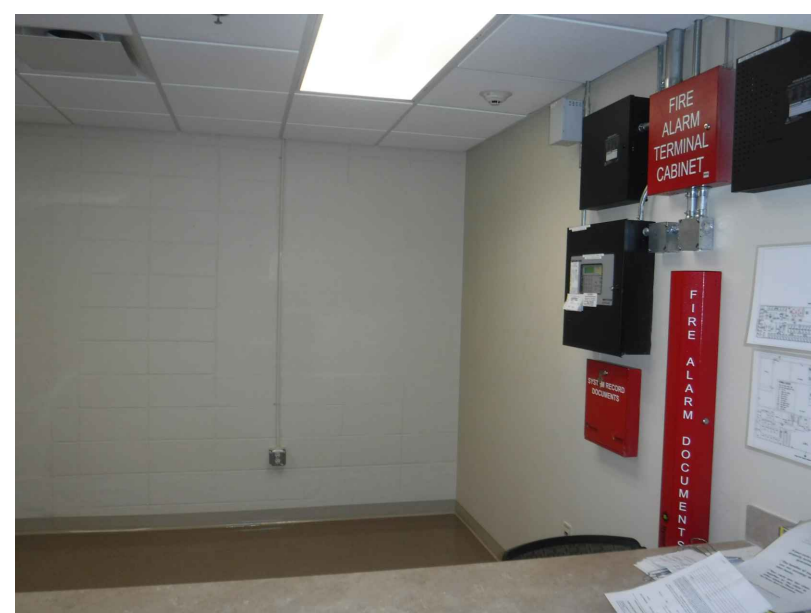
EXISTING F.A. EQUIPMENT TO REMAIN IN NEW SECURITY SYSTEM COMMAND CENTER
