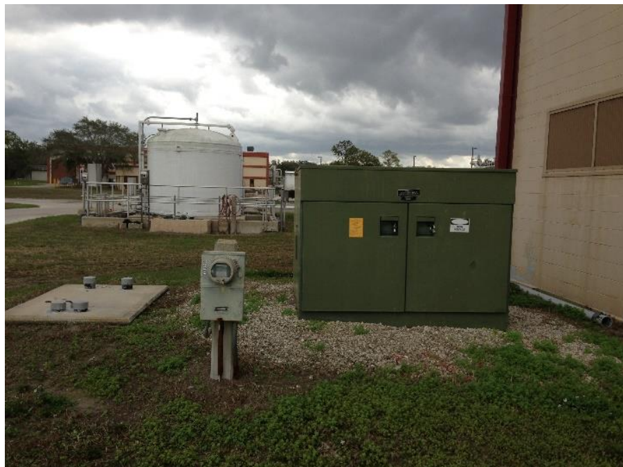
Figure 2.2 OUC 600A Switch "A" Solids Building
