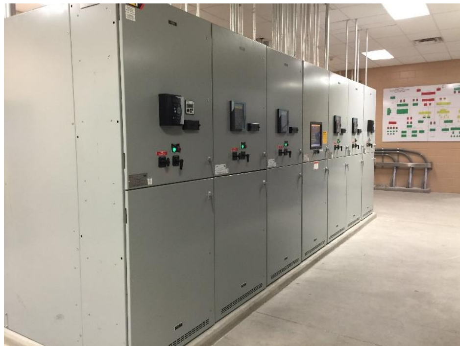
Figure 3.4 Existing 12,470 Volt Generator Switchgear
