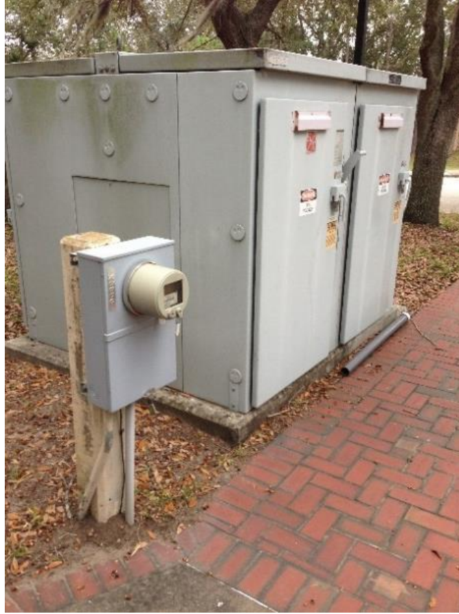
Figure 2.4 OUC 600A Switch "B" Admin Building
