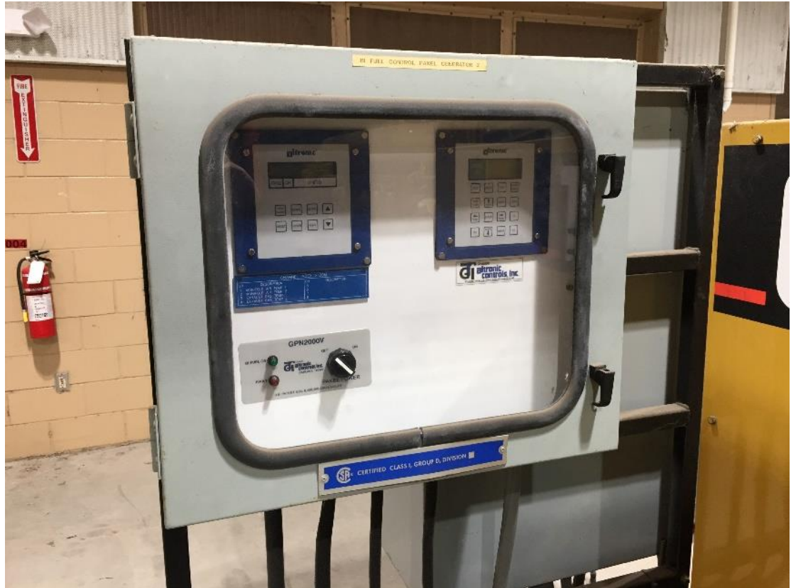
Figure 3.7 Generator Dual Fuel Control Panel
