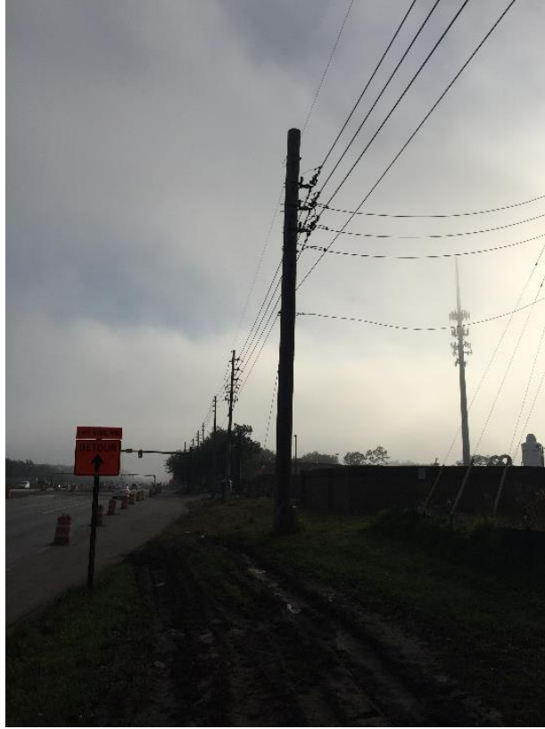
Figure 2.5 Common OUC Utility Pole for Service "A" & "B"
