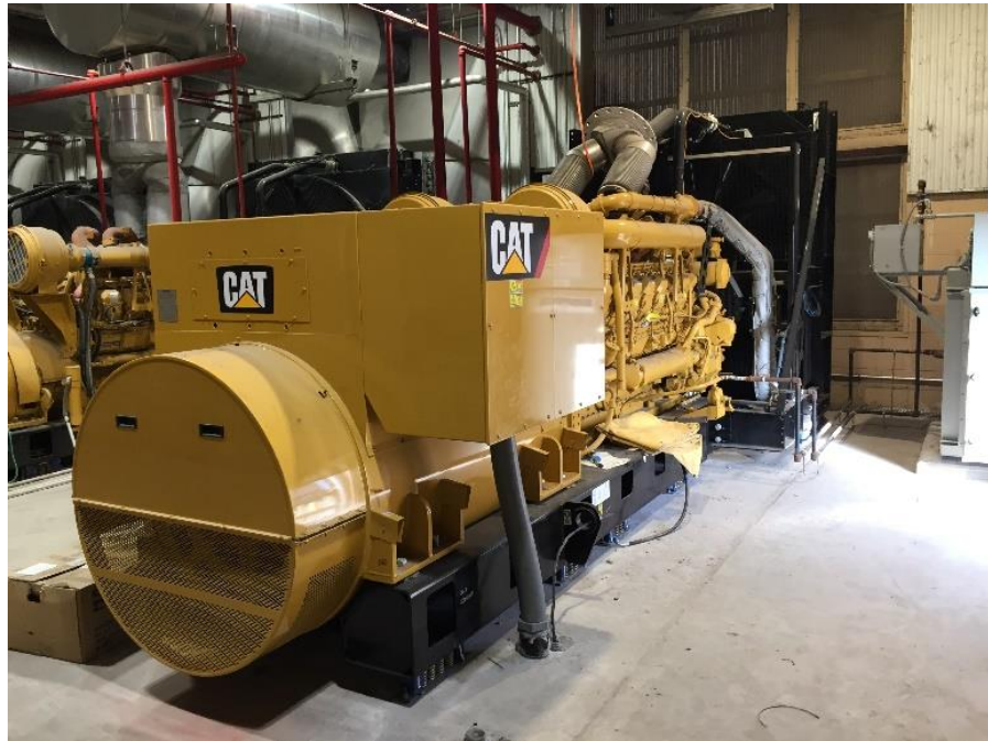
Figure 3.2 New 2500 KW Generator (Installed During Phase V Construction)
