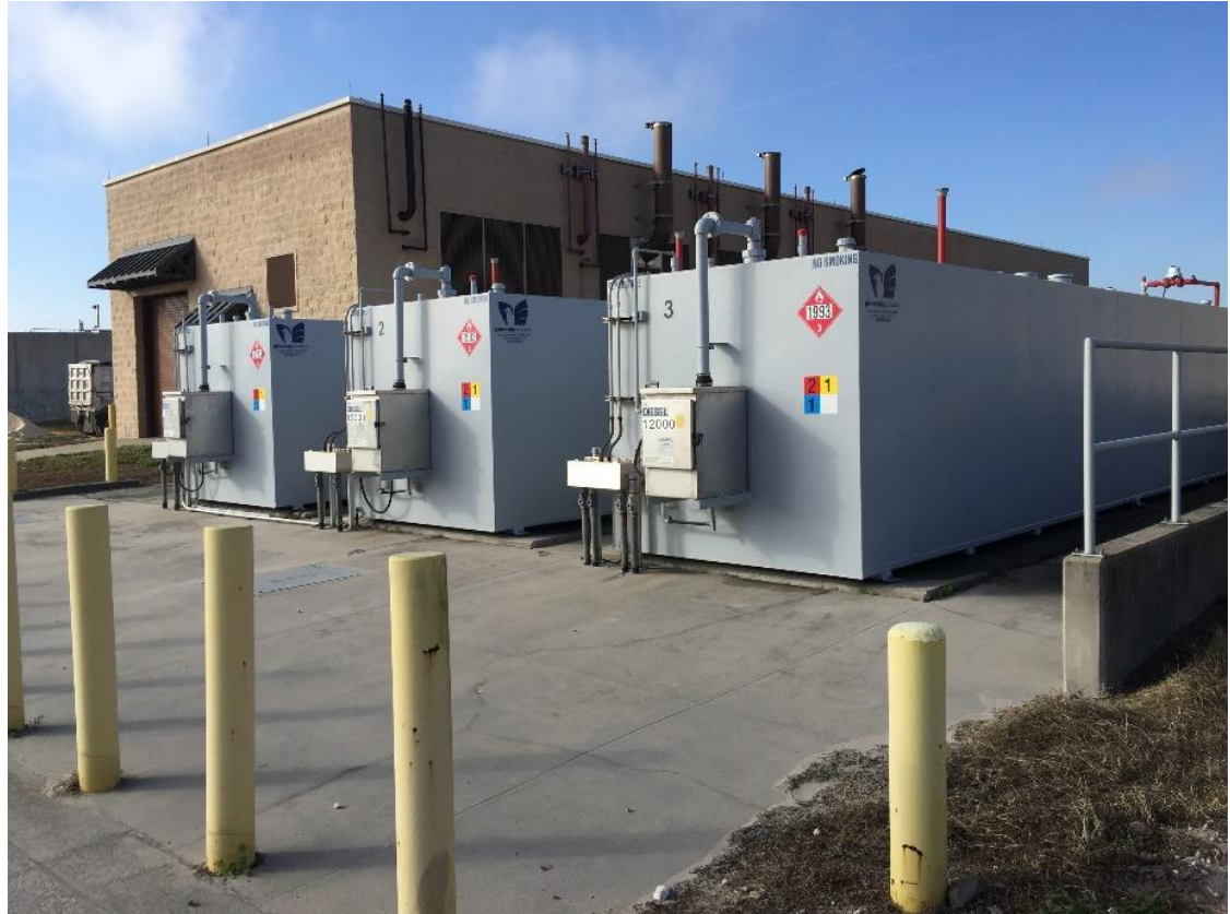
Figure 3.8 Existing (3) 12,000 Gallon Fuel Tanks
