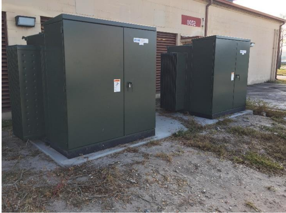
Figure 2.6 Typical A & B Service Transformers/Switch
