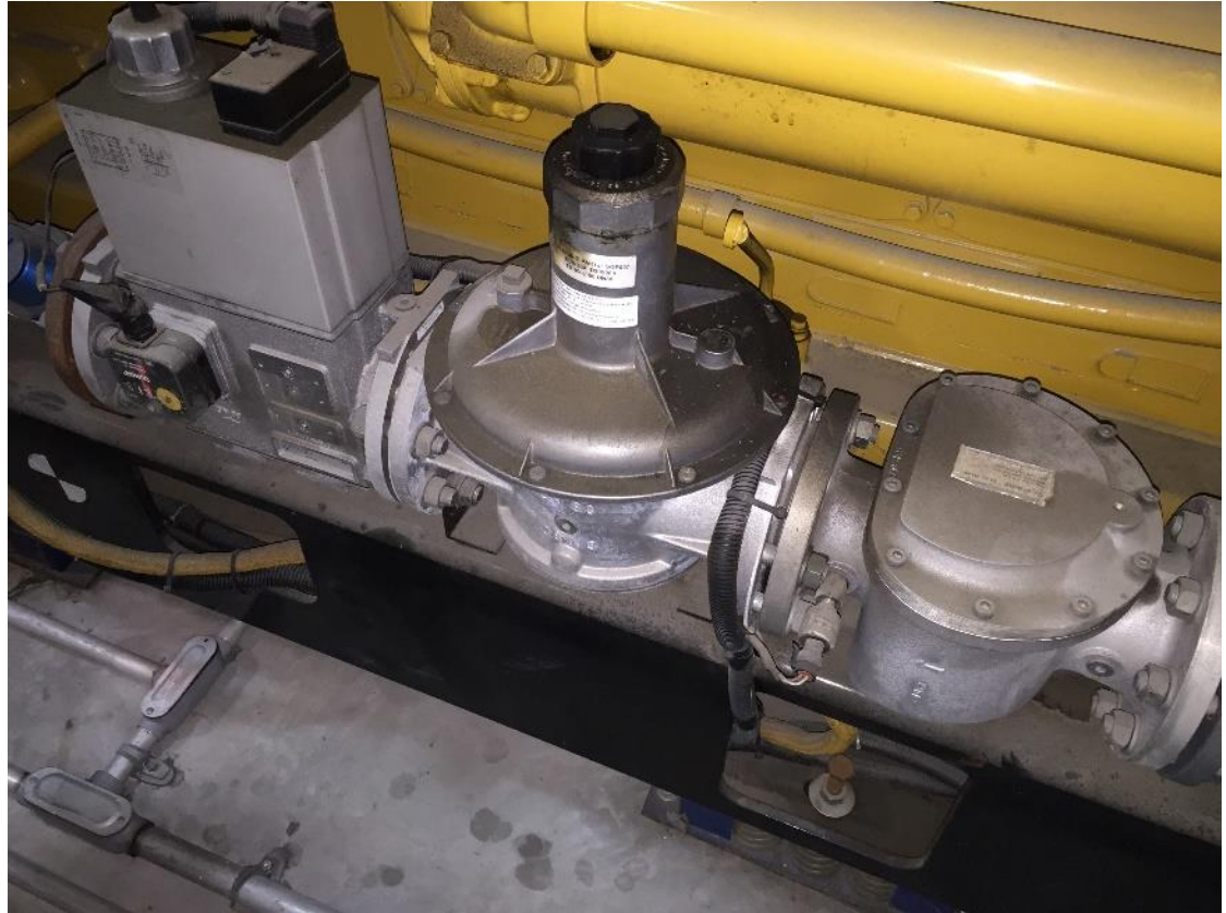
Figure 3.5 Generator Dual Fuel Natural Gas Trane at Generator
