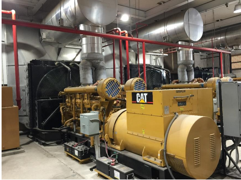
Figure 3.1 Existing Dual Fuel 2250 KW Generator System
