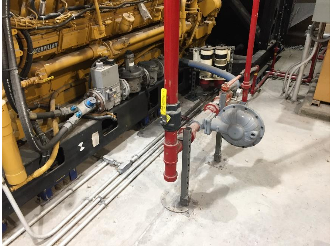
Figure 3.6 Dual Fuel Regulator and Generator Piping
