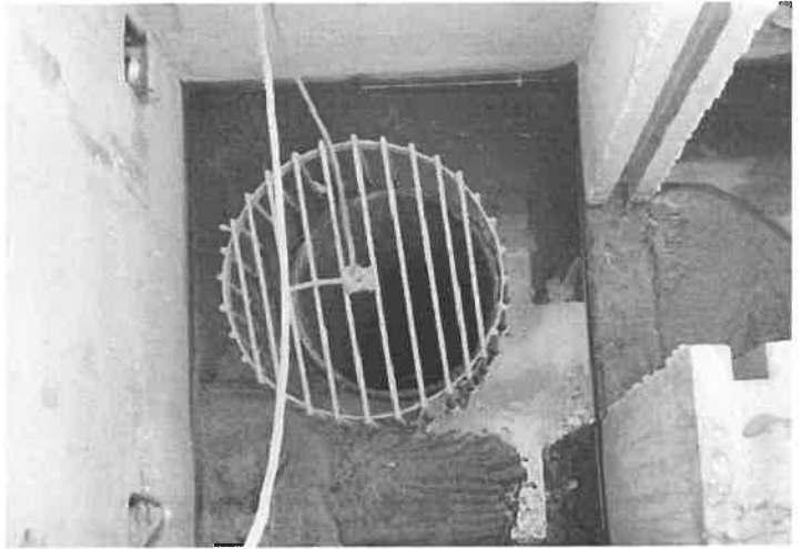
04. Interior closeup view of well head.
