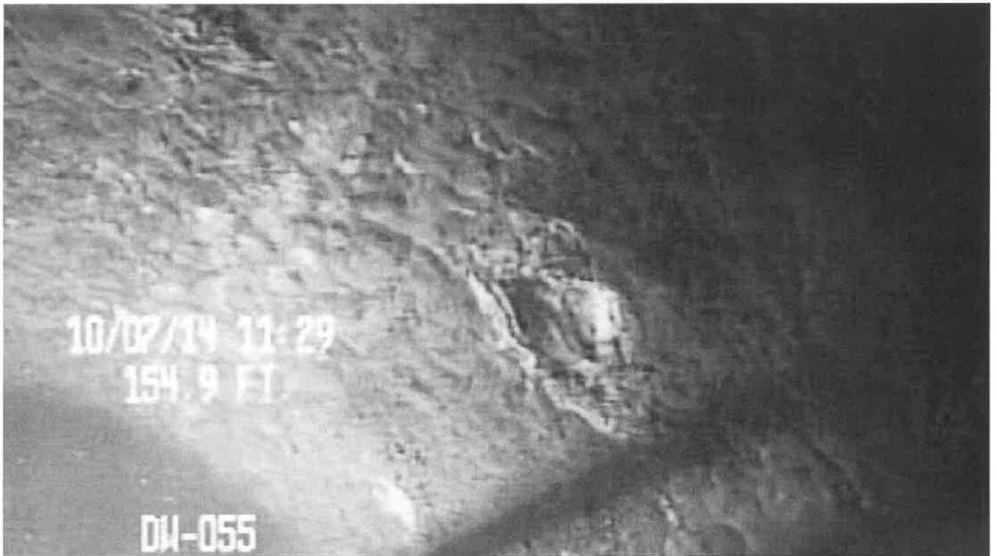
18. Encrusted casing at 154.9ft-2014
