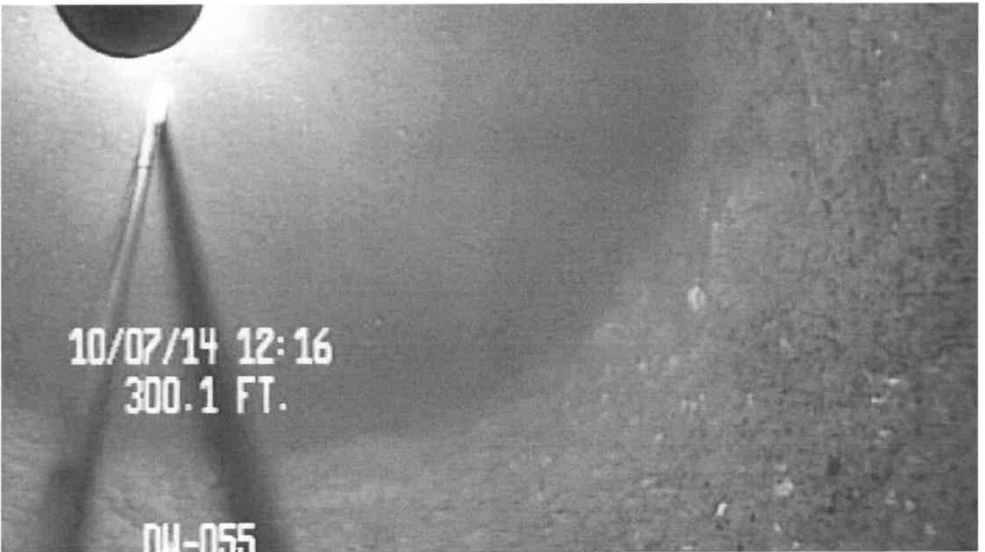
20. Encrusted casing at 300ft-2014
