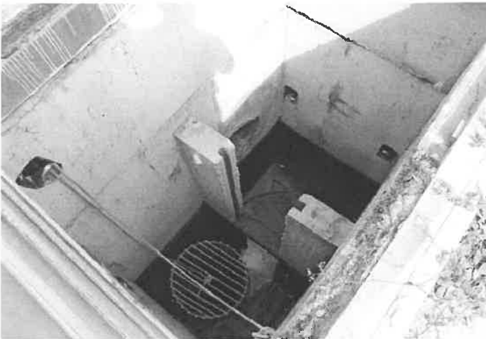
03. Interior view of structure showing well head with debris screen, weir and inflow pipe.
