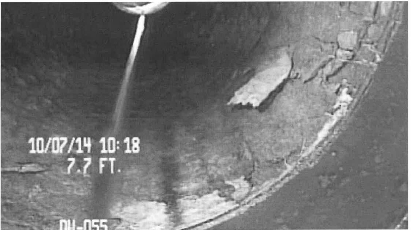
02. Slaking at top of well casing at 7.7 ft depth - 2014
