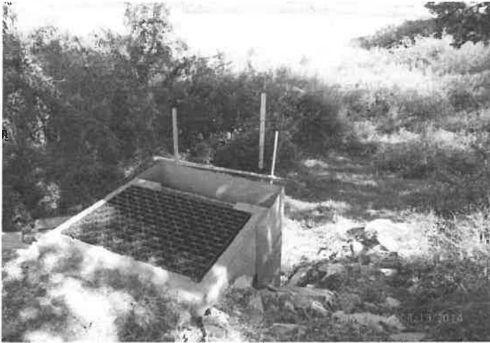
05. Concrete inflow device with fiberglass skimmer and staff gage beyond
