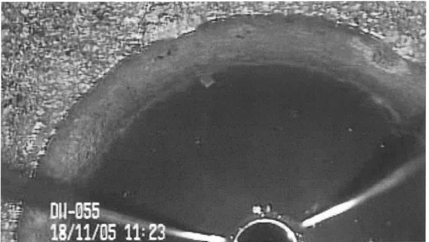
09. Slaking at water level-24.7ft-2011
