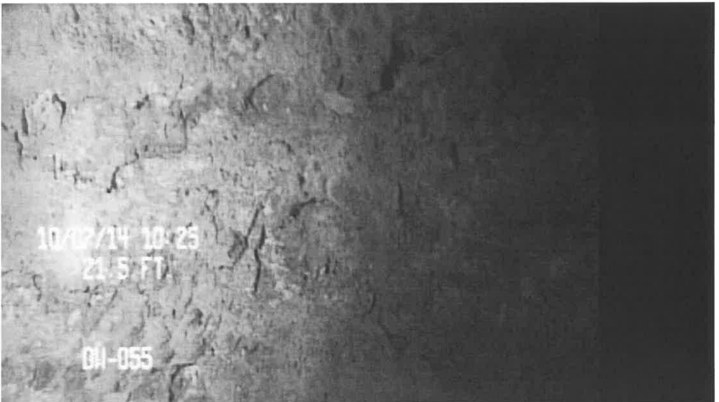
12. Pitting & slaking at 21.5ft-2014
