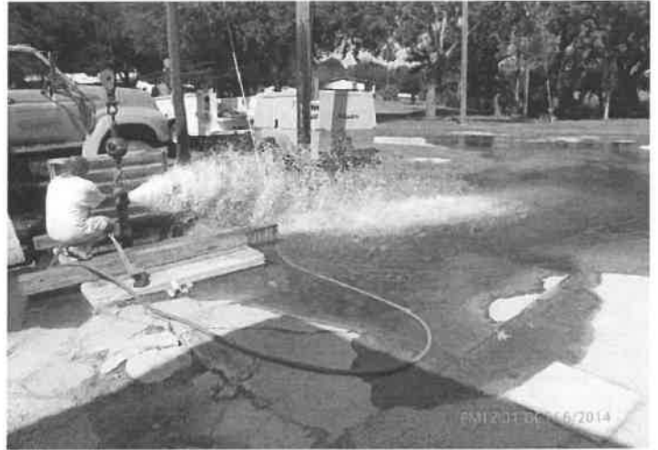
10. Additional view of discharge during cleaning
