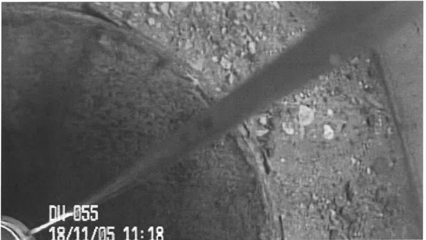
01. Slaking at top of well casing at 7.7 ft depth - 2011
