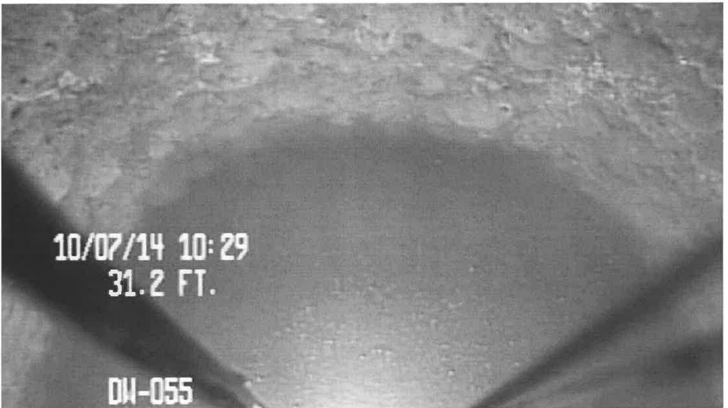
14. Encrusted casing at 31.2ft-2014
