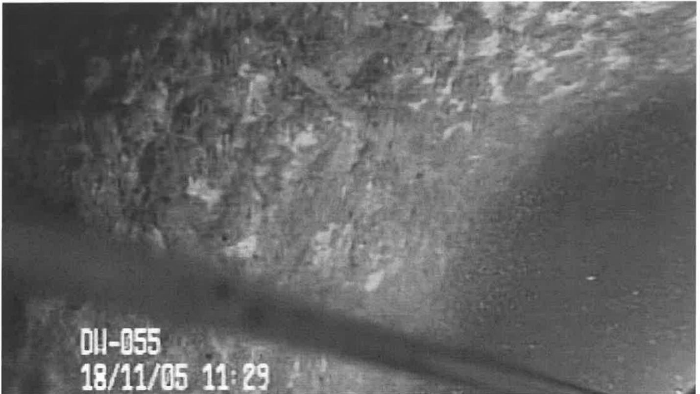
15. Encrusted casing at 60.7ft-2011
