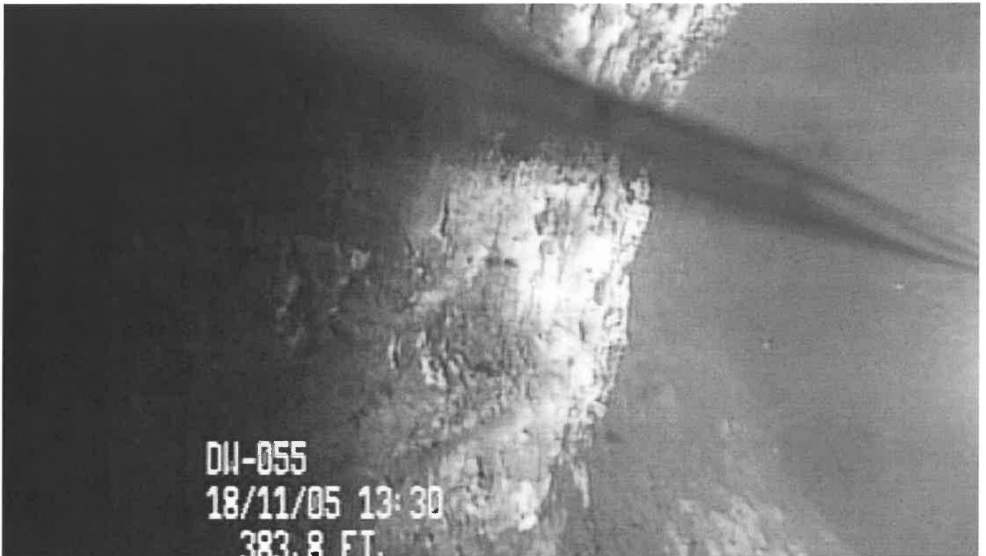
21. Bottom of casing - estimated at 383.8ft-2011
