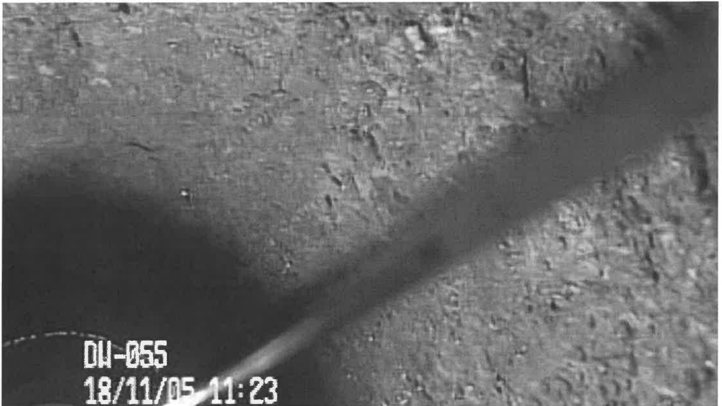
11. Pitting and slaking at 21.5ft-2011
