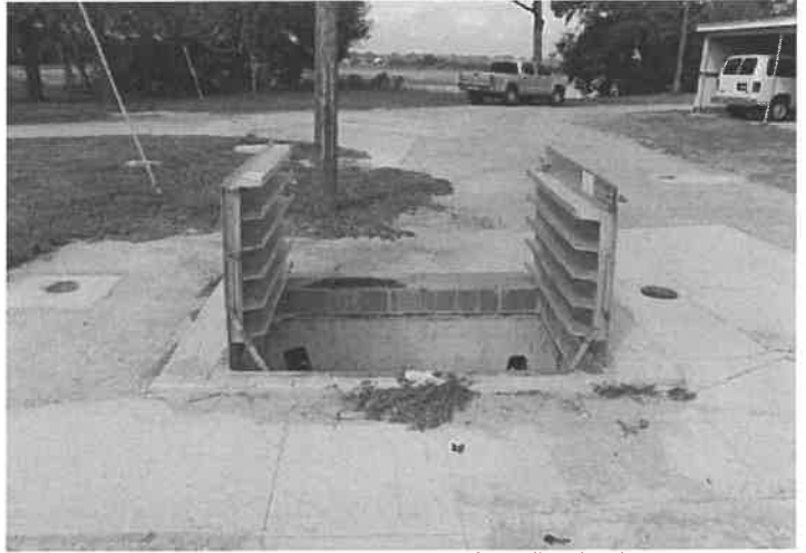
02. View of dual aluminum hatch covers for well and weir structure.
