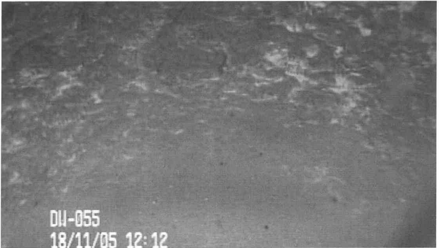
17. Encrusted casing at 155.4ft-2011
