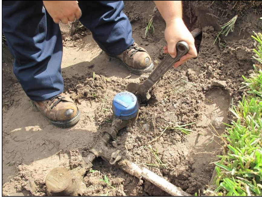
Figure 16. Loosening Meter coupling
