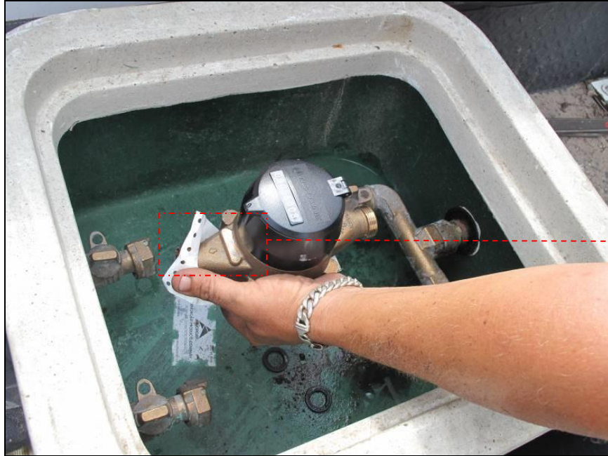
Figure 30. Arrow on meter indicates direction of flow
