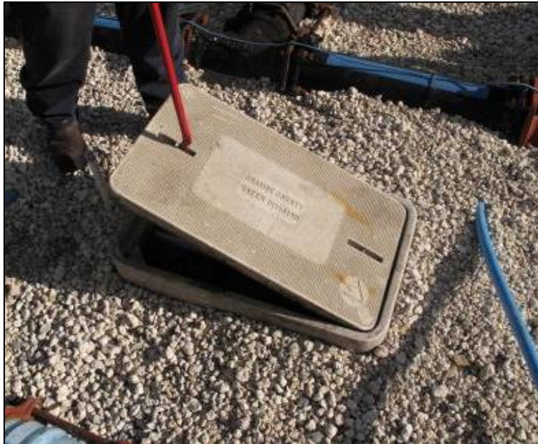
Figure 2. Meter box lid removal
