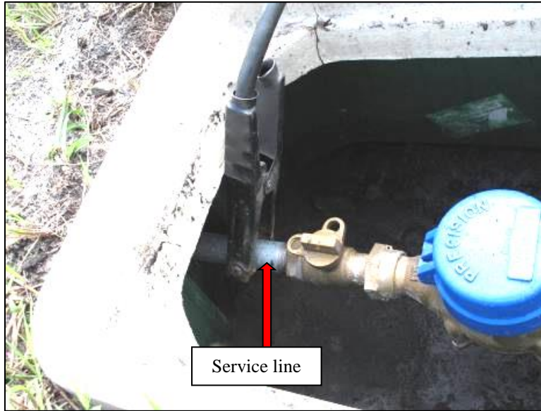
Figure B. One end of jumper cable clamped on service line
