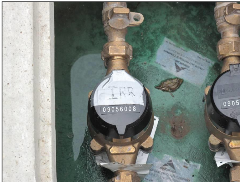
Figure 45. Labeled irrigation meter
