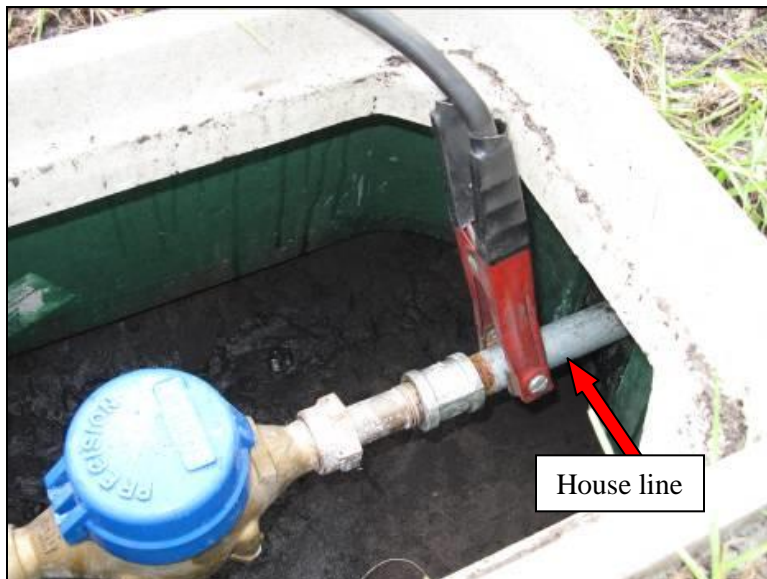
Figure 3. The other end of jumper cable clamped on house line
