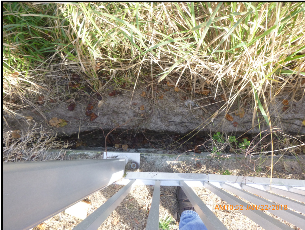
Exhibit 14. Soil Pulling Away From Downslope Side of Wall (1/22/2018)
