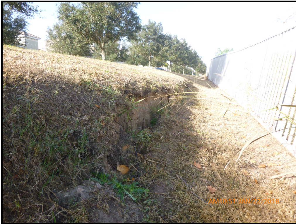
Exhibit 13. Close up of Shear Failure Scarp Looking West (1/22/2018)
