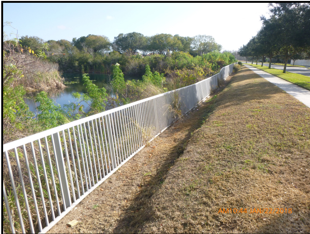
Exhibit 12. View of Subsidence Along Retaining Wall Fence Looking East (1/22/18)
