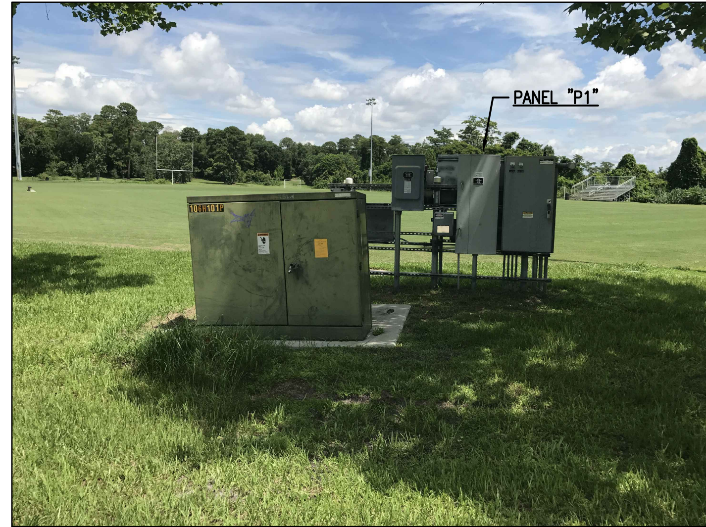
LOCATION OF PANEL "P1" AT OUC TRANSFORMER
