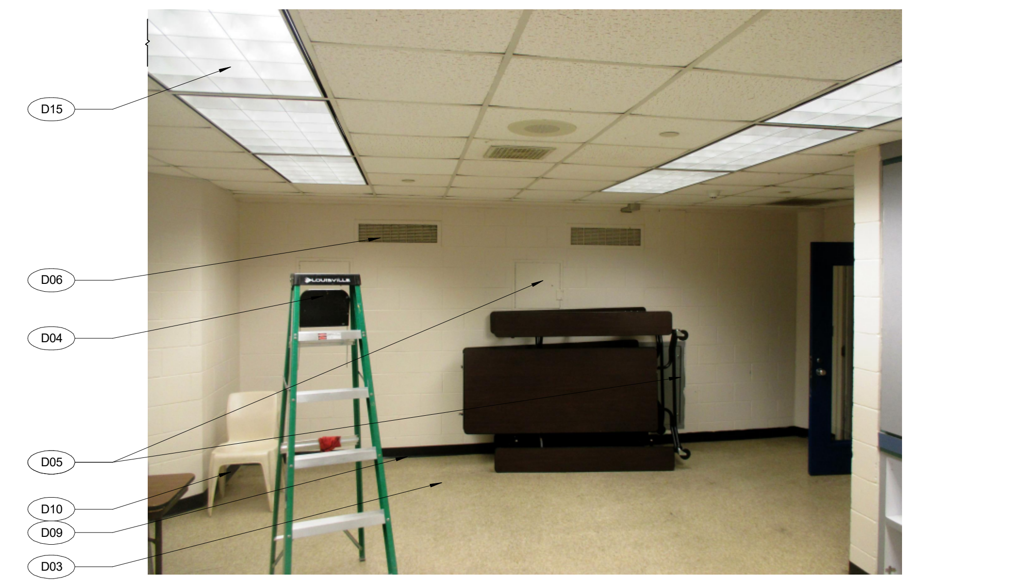
5 AD102 EXISTING PHOTO AT LEVEL 4 CLASSROOM "C" CHASE WALL (TYP OF LEVEL 6) SCALE: 1/4" = 1'-0"
