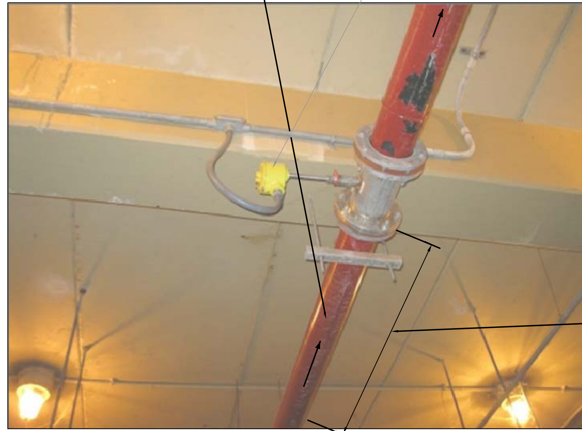
GAS GOING TO WASTE GAS BURNERS
