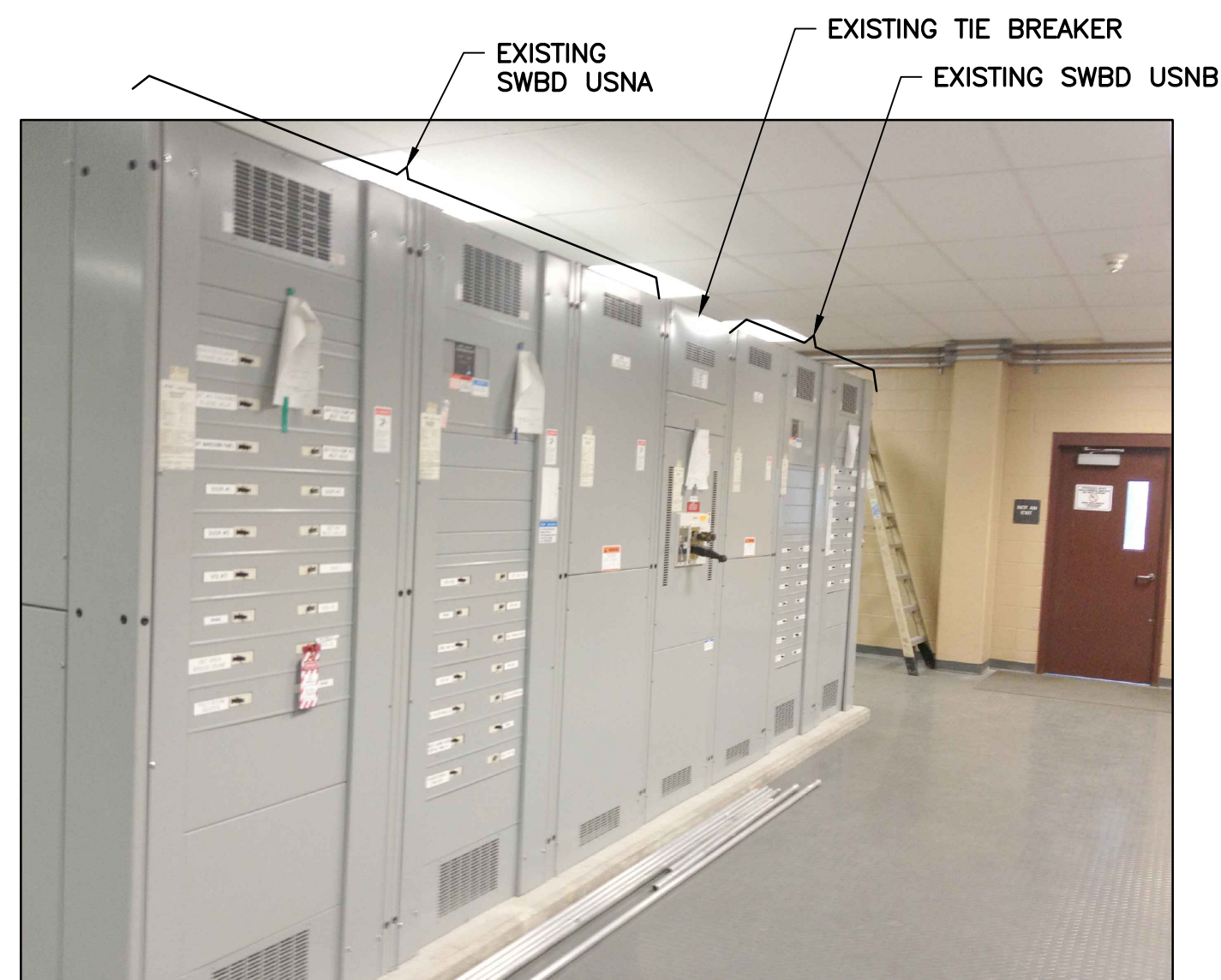
EXISTING SWBD 'USNA' & 'USNB' OVERALL EQUIPMENT FRONT VIEW (DEWATERING BUILDING ELECTRICAL ROOM) N.T.S.
