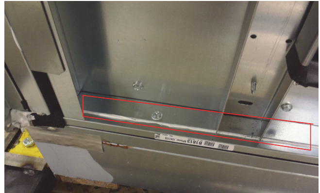
Figure 11. COU panel and filter racks
