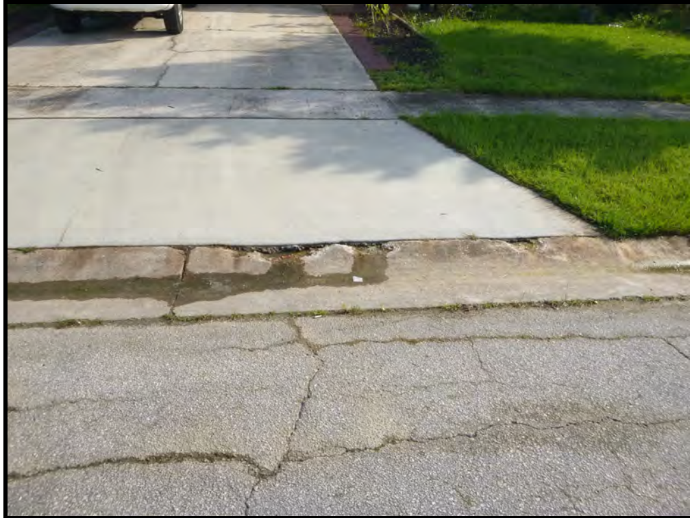
Photo #3. Seepage on Jepson Street
