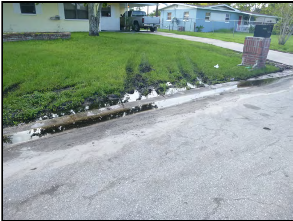
Photo #4. Seepage on Roberta Avenue
