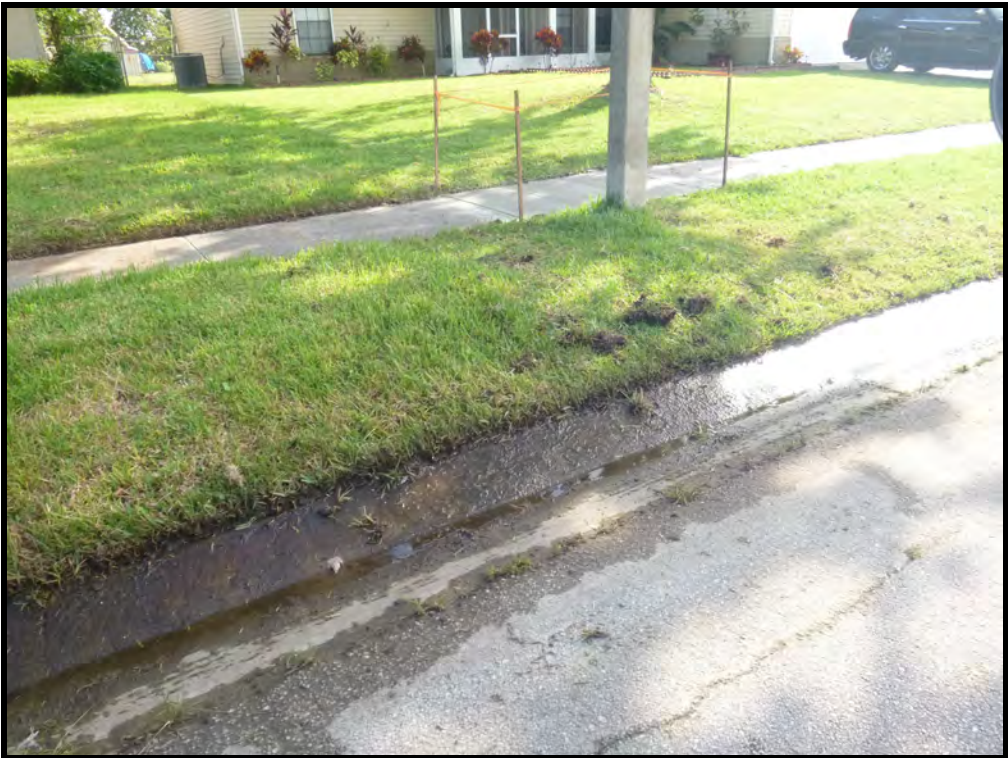
Photo #2. Seepage on Bridlewood Avenue
