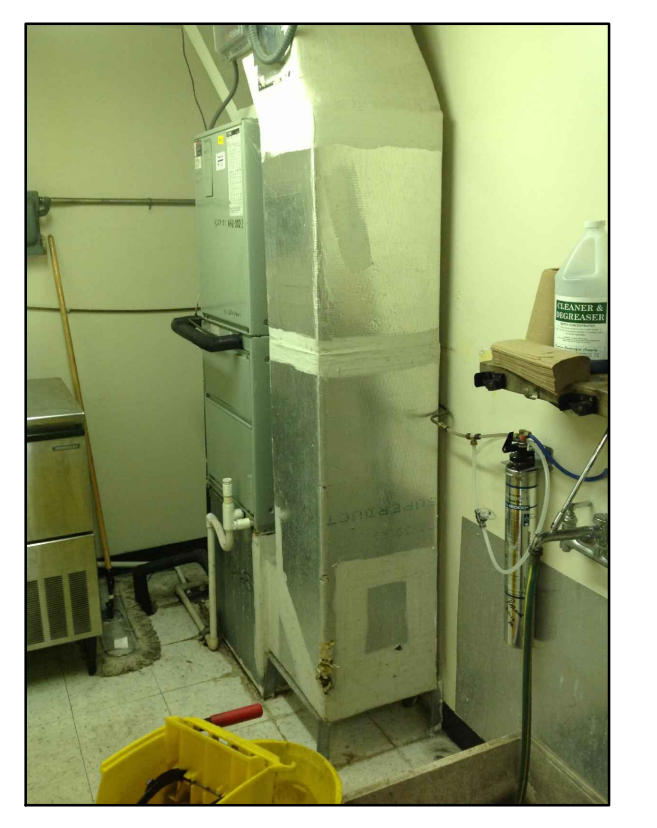
AIR HANDLING UNIT AHU-2 TO BE REMOVED AND REPLACED
