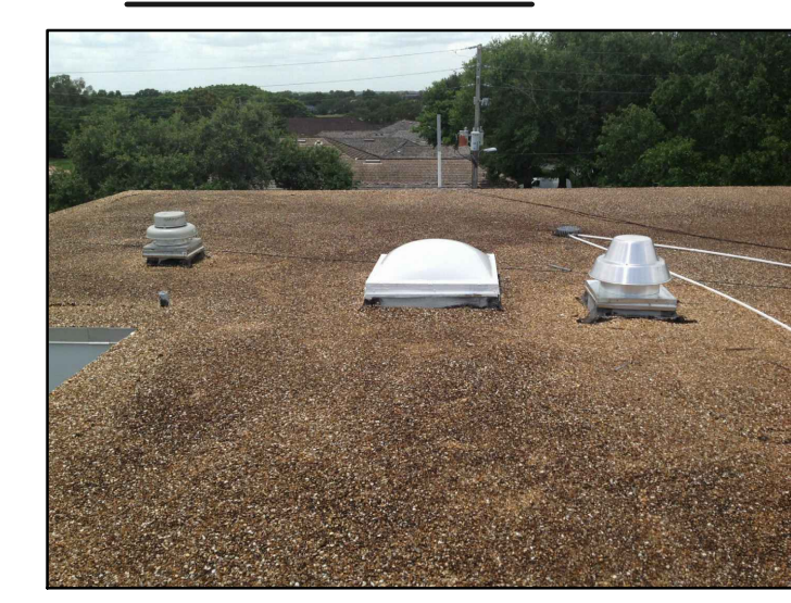
EXHAUST FANS EF-2 & EF-4 TO BE REMOVED AND REPLACED
