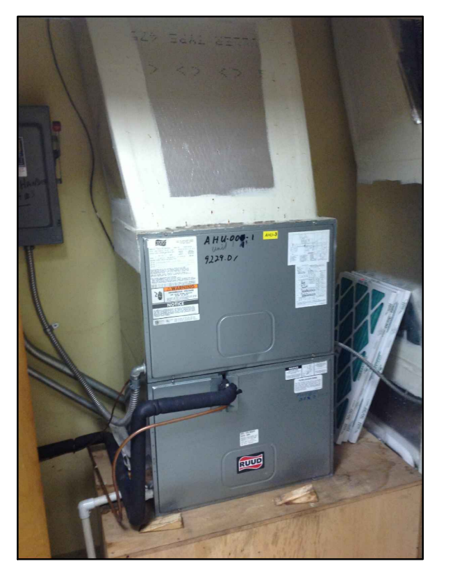
AIR HANDLING UNIT AHU-3 TO BE REMOVED AND REPLACED
