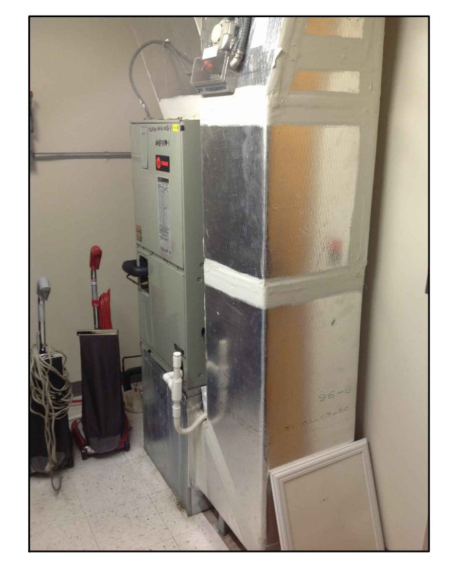
AIR HANDLING UNIT AHU-1 TO BE REMOVED AND REPLACED
