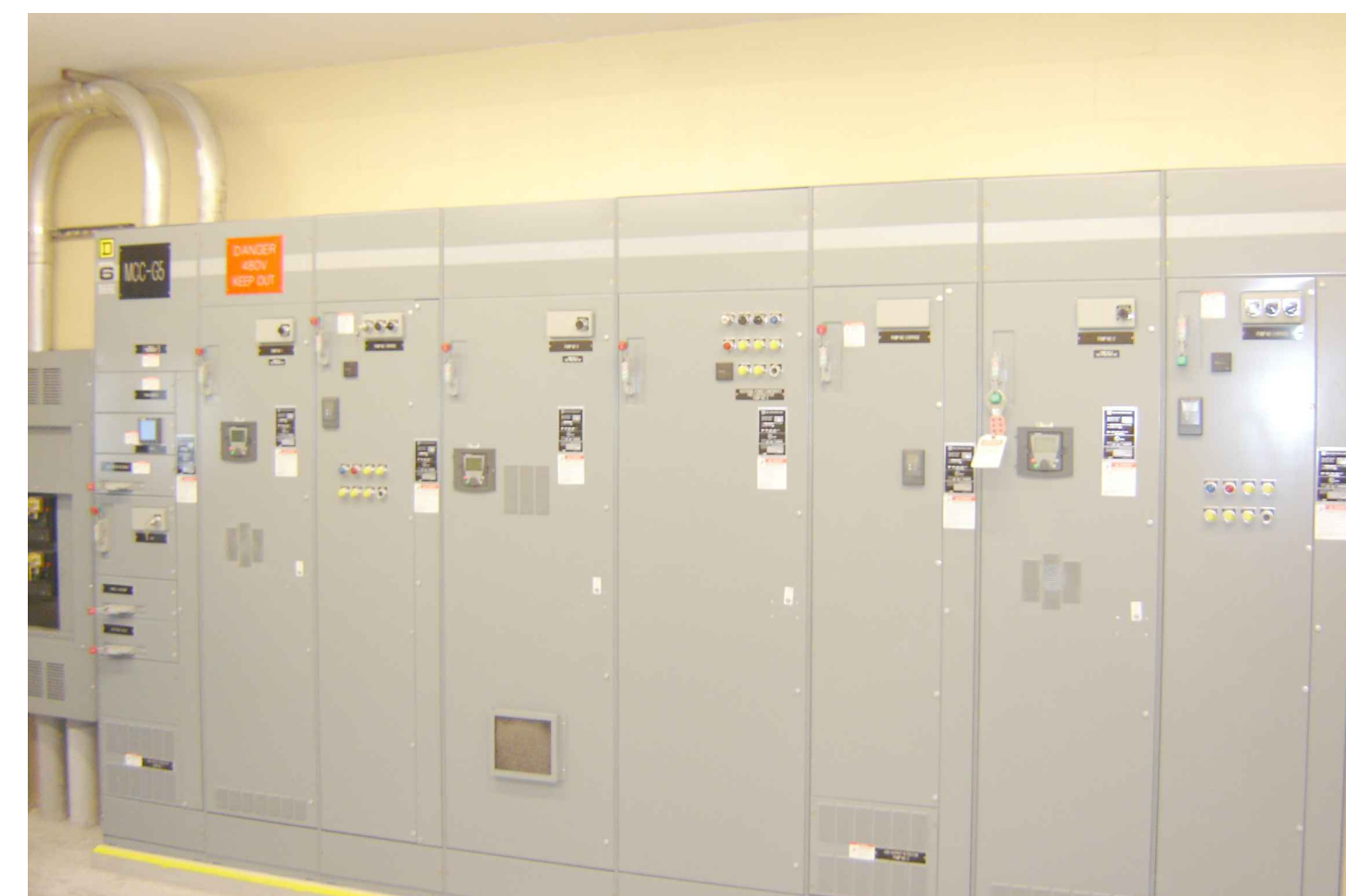
3 FIGURE NO. 1 - MCC-G5 FRONT VIEW E-6 N.T.S.
