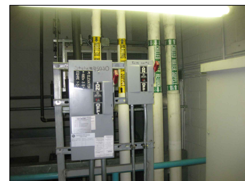
EXISTING CHILLED WATER AND HOT WATER PIPING TO BE REMOVED IN IT'S ENTIRETY (AHU-29 BEHIND PIPING)
