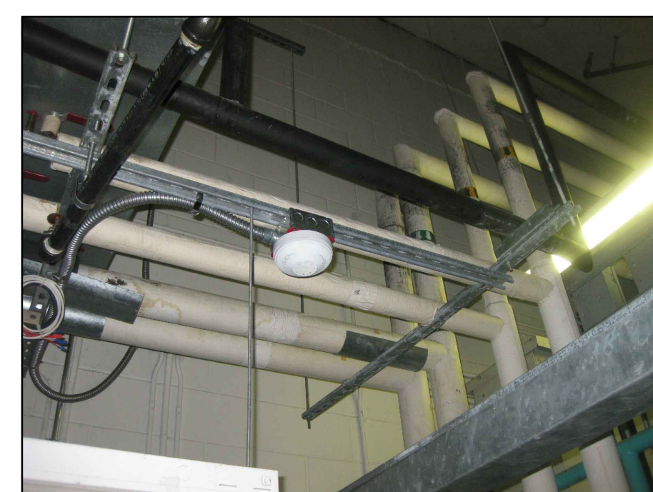
EXISTING CHILLED WATER, HOT WATER PIPING AND CONDENSATE PIPING TO BE REMOVED IN IT'S ENTIRETY (TO AHU-29 & AHU-30)
