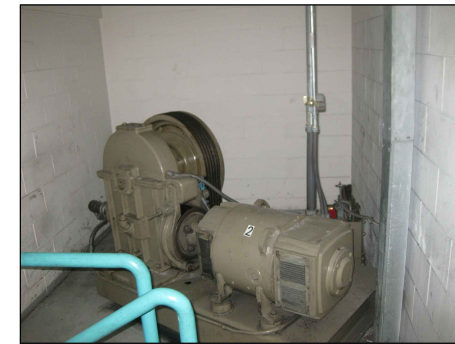
EXISTING ELEVATOR MOTOR TO BE REMOVED AND REPLACED
