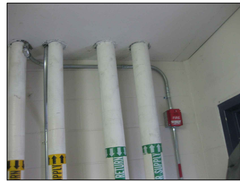
EXISTING CHILLED WATER AND HOT WATER PIPING THROUGH FLOOR TO BE REMOVED IN IT'S ENTIRETY (ROOF ELEV. VESTIBULE TO 2ND PLATFORM)
