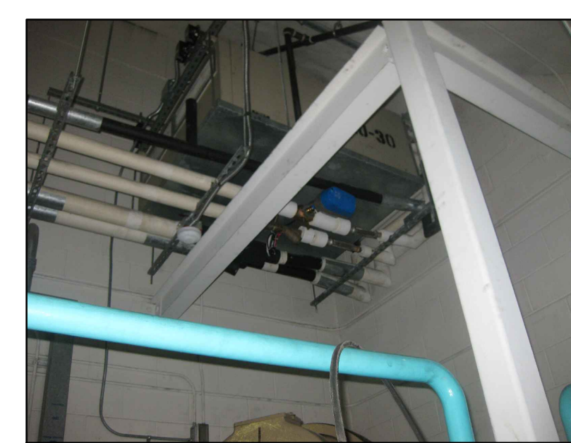
EXISTING AHU-30 AND ALL ASSOCIATED CHILLED WATER, HOT WATER AND CONDENSATE DRAIN PIPING TO BE REMOVED IN IT'S ENTIRETY
