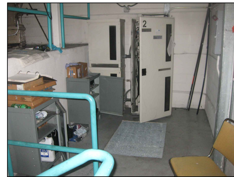
EXISTING ELEVATOR CONTROLLERS TO BE REMOVED AND REPLACED
