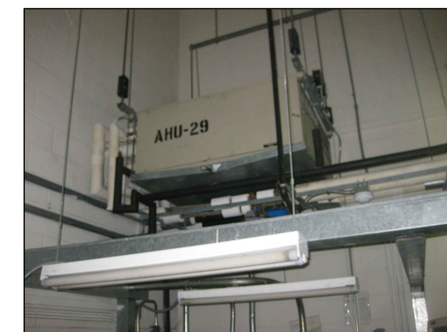
EXISTING AHU-29 AND ALL ASSOCIATED CHILLED WATER, HOT WATER AND CONDESANTE DRAIN PIPING TO BE REMOVED IN IT'S ENTIRETY
