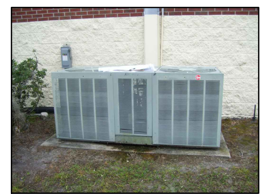
HEAT PUMP UNIT HP-3
