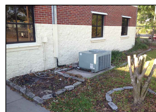
HEAT PUMP UNIT HP-1
