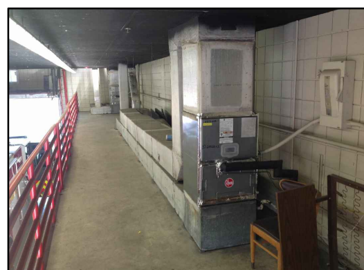
AIR HANDLING UNIT AHU-2
