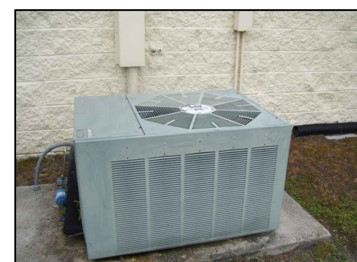
HEAT PUMP UNIT HP-2
