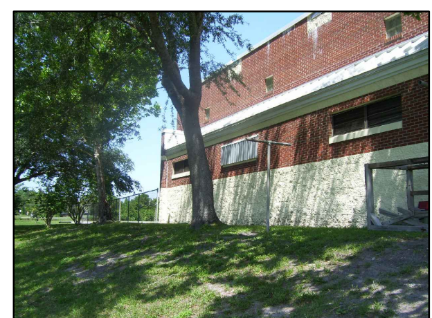
APPARATUS BAY O.A. INTAKE LOUVERS
