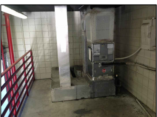
AIR HANDLING UNIT AHU-1
