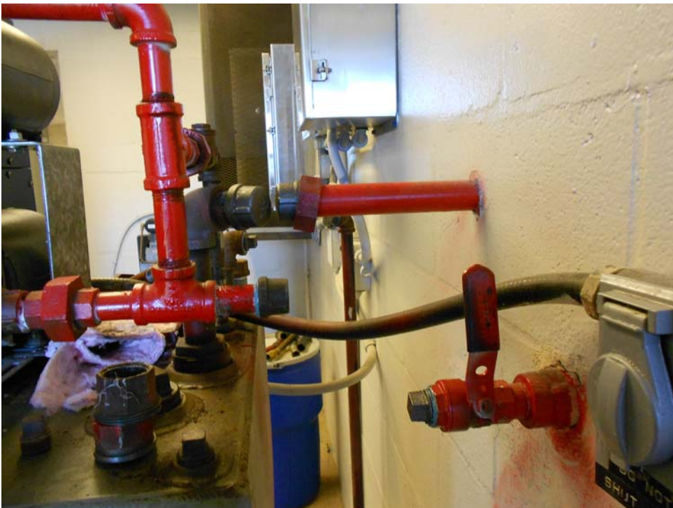
Photo of capped product piping 10/31/12
