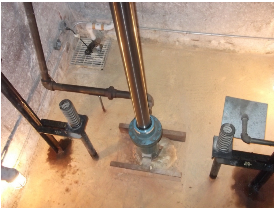
Below: Pit equipment to be retained, refurbished and painted. Elected General Contractor to ensure the existing Sump/Pump complies with local plumbing codes
