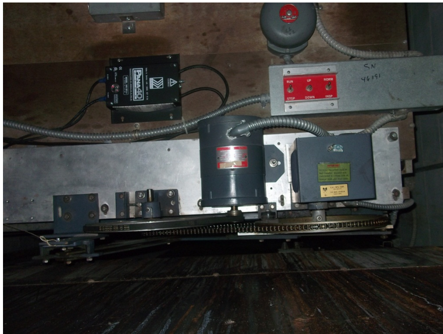
Below: Car top equipment and car side door equipment to be replaced; to include, door operator, clutch w/restrictor, inspection station, and code compliant escape hatch.
