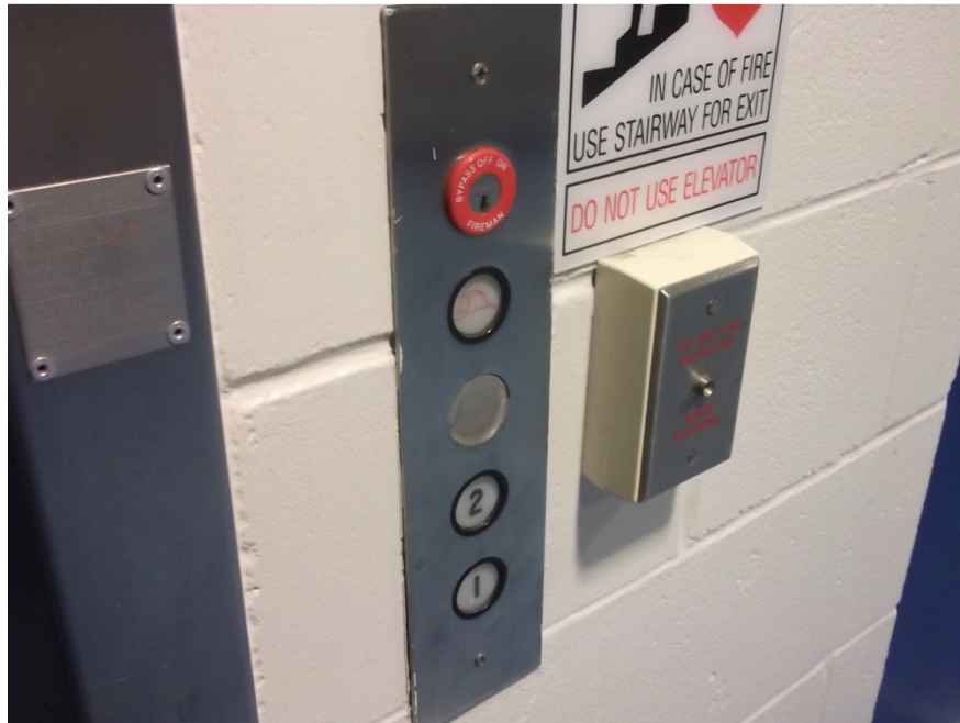
Above: Hall Fixtures will be replaced, fire emergency signage to be engraved in new fixture plate.
