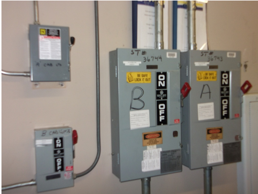
Above: While the disconnects may be code compliant, when performing a modernization it is always the best time to replace the disconnects to ensure longevity of the entire system.
