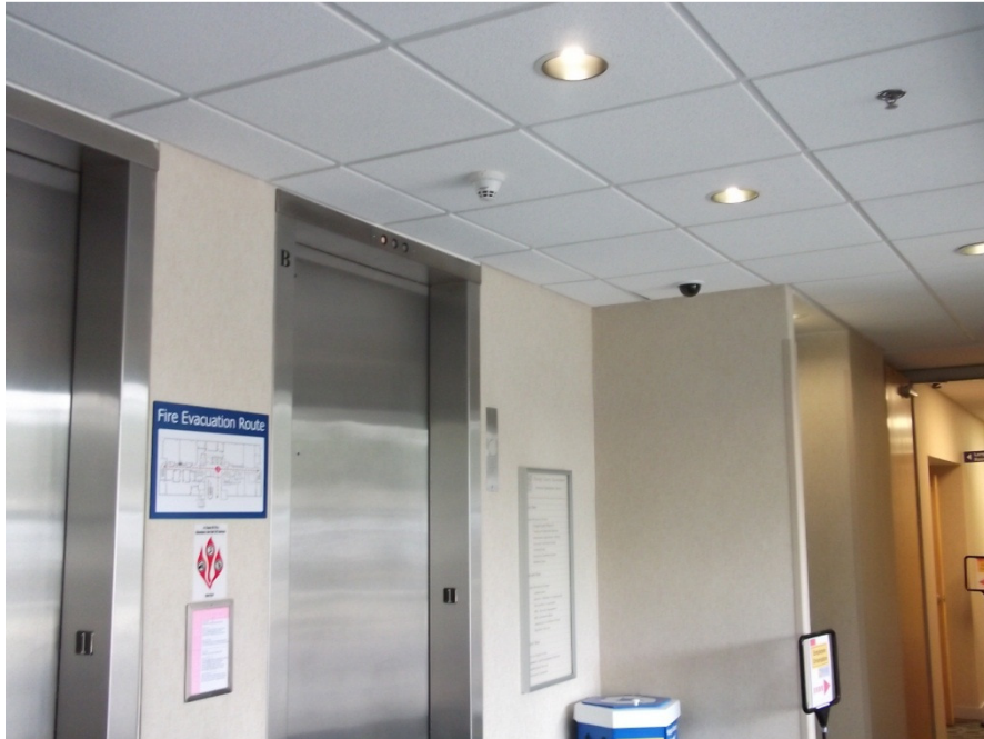
Above: Main lobby floor has code compliant smoke head and sprinkler.
