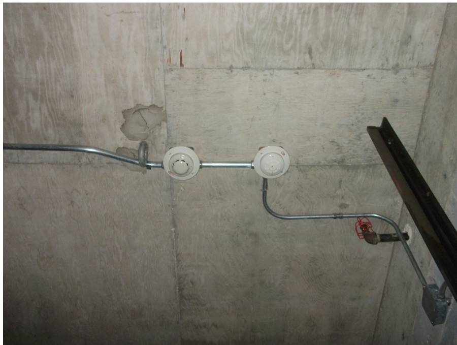
Below: Top of shaft is sprinkled, shunt trip currently installed and must remain. Shaft requires venting.
