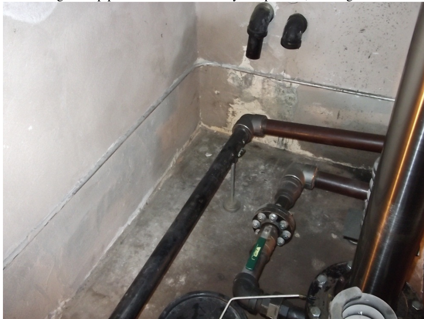
Below: Old underground pipe should be cut off fully and patched, existing oil line to be retained
