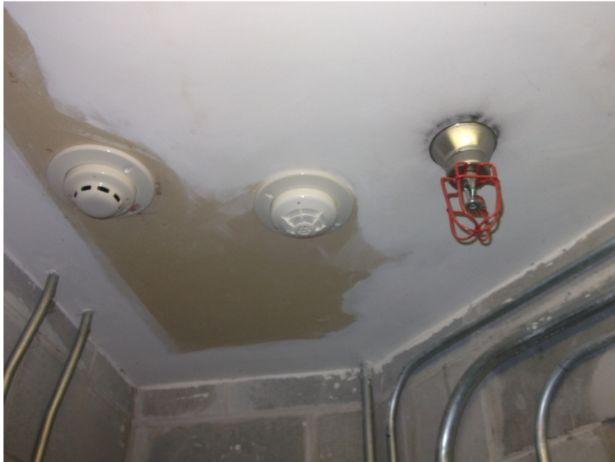
Above: Machine room has smoke, heat and sprinkled.
