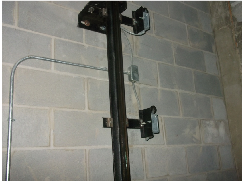
Above: Limit switches will be replaced during the modernization.
