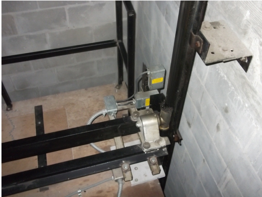
Above: Slide guide inserts to be replaced new.
