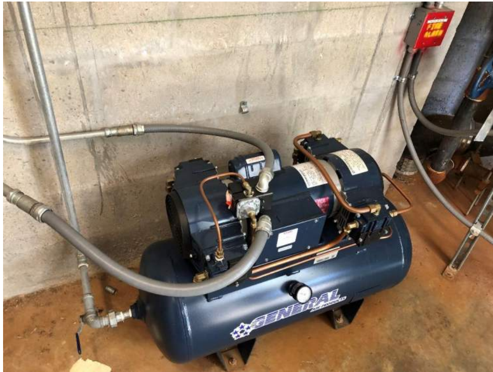
Photo #6 – Horizontal Compressed Air System for Dry-Pipe Valves – HUB 2
