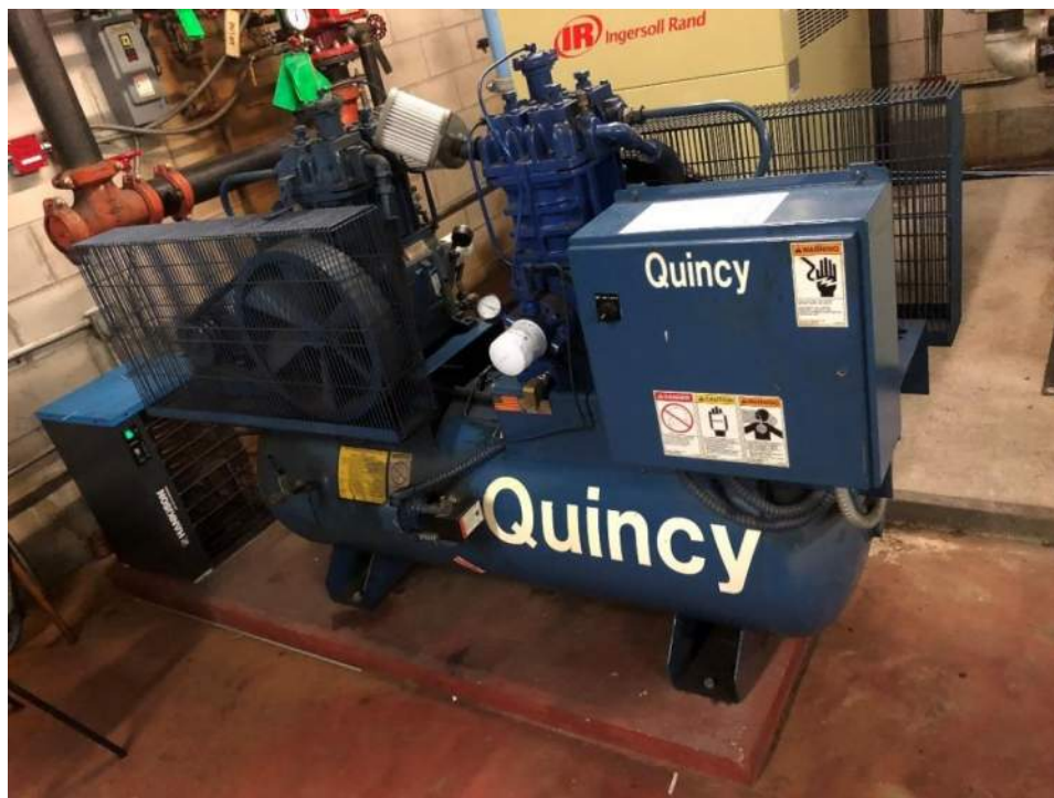
Photo #3 – Plant Compressed Air System serving Dry-Pipe Valves
