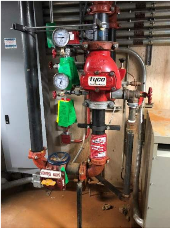
Photo #13 – Dry-pipe Assembly in Tunnel Level
