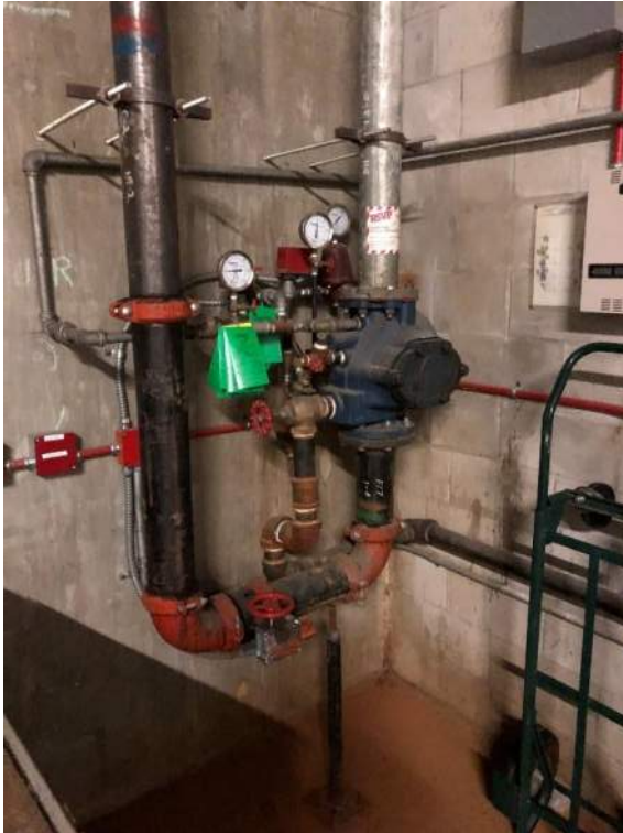
Photo #1 – Older Style Dry-Pipe Valve
