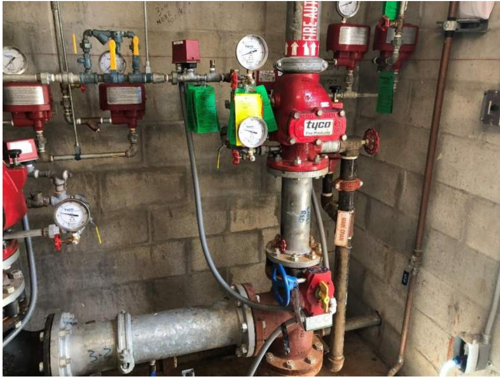
Photo #8 – Dry-Pipe Valve – HUB 2
