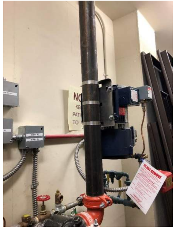
Photo #14 – Riser Mounted CA System
