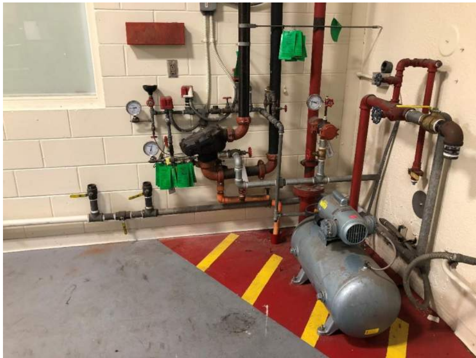
Photo #12 – Older Style Dry-pipe Assembly
