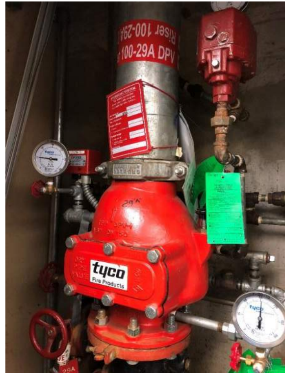
Photo #2 – Newer Style Dry-Pipe Valve
