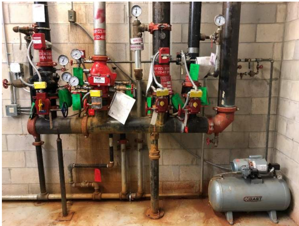
Photo #9 – Dry-Pipe Valve Assembly from Wet-Pipe Header
