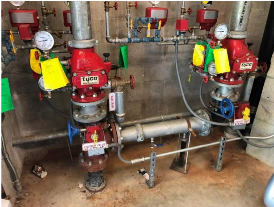
Photo #5 – Dry-Pipe Valves – HUB 1
