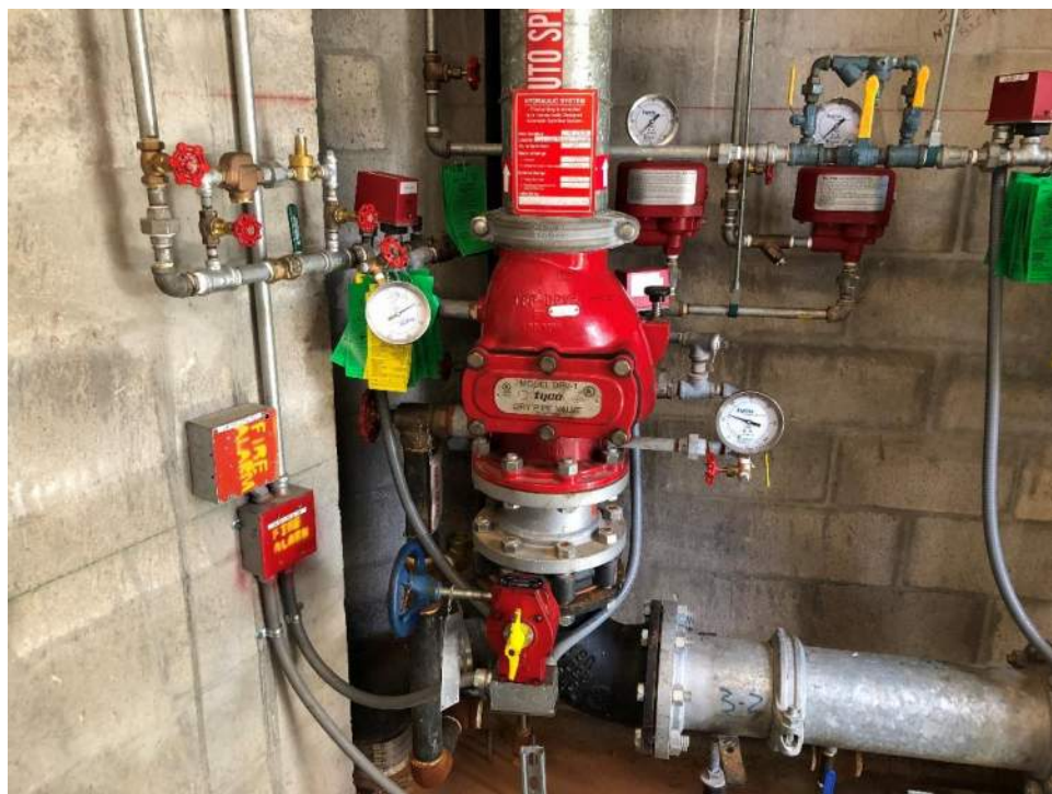
Photo #7 – Dry-Pipe Valve – HUB 2
