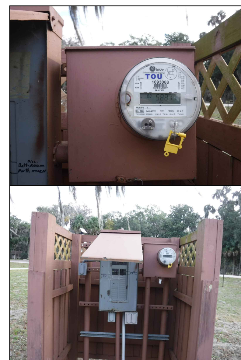
EXISTING NEMA 3R ELECTRICAL PANEL "E" EXISTING METER No. 1093068
