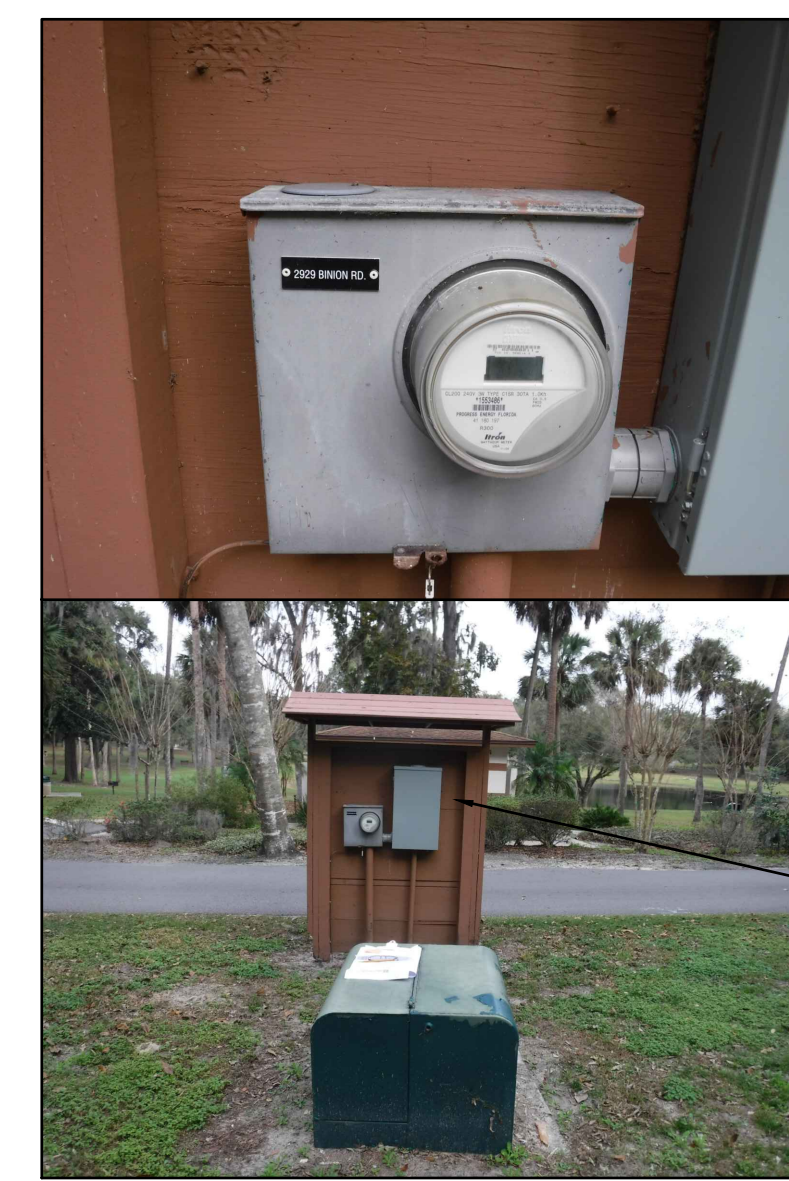
EXISTING NEMA 3R ELECTRICAL PANEL "B" EXISTING METER No. 1553486.
