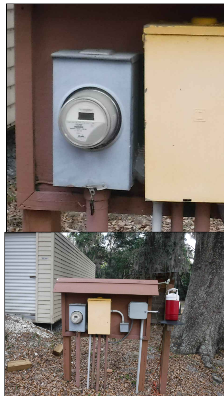
EXISTING NEMA 3R ELECTRICAL PANEL "d" EXISTING METER No. 1553498.
