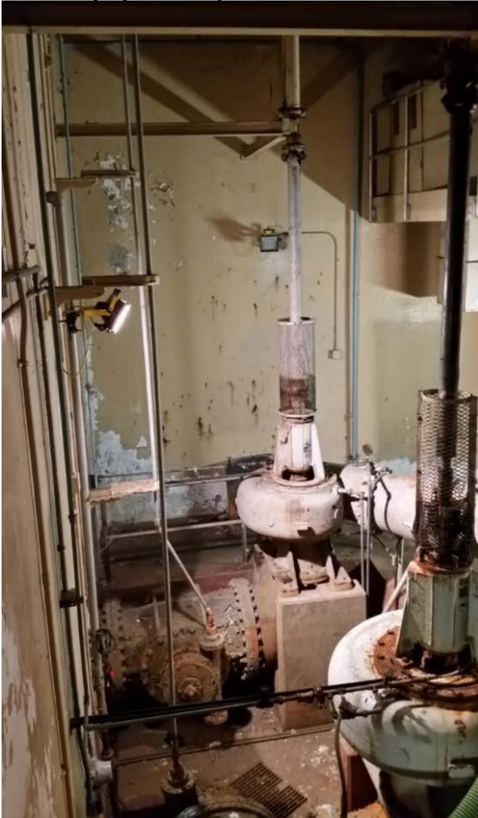
6. North pump room looking west
