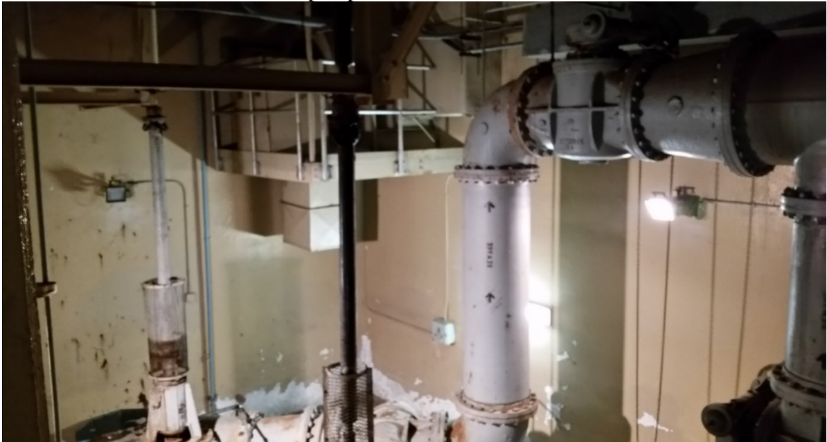
4. Elevated view in the north pump room
