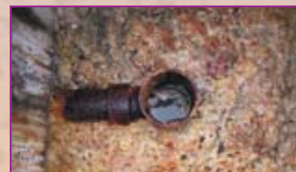
Oil and grease accumulation in a poorly maintained grease removal device.
