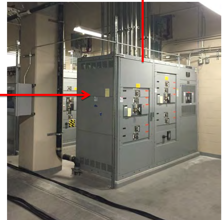
Fig. 2.3 Typical 3000A Switchboard
