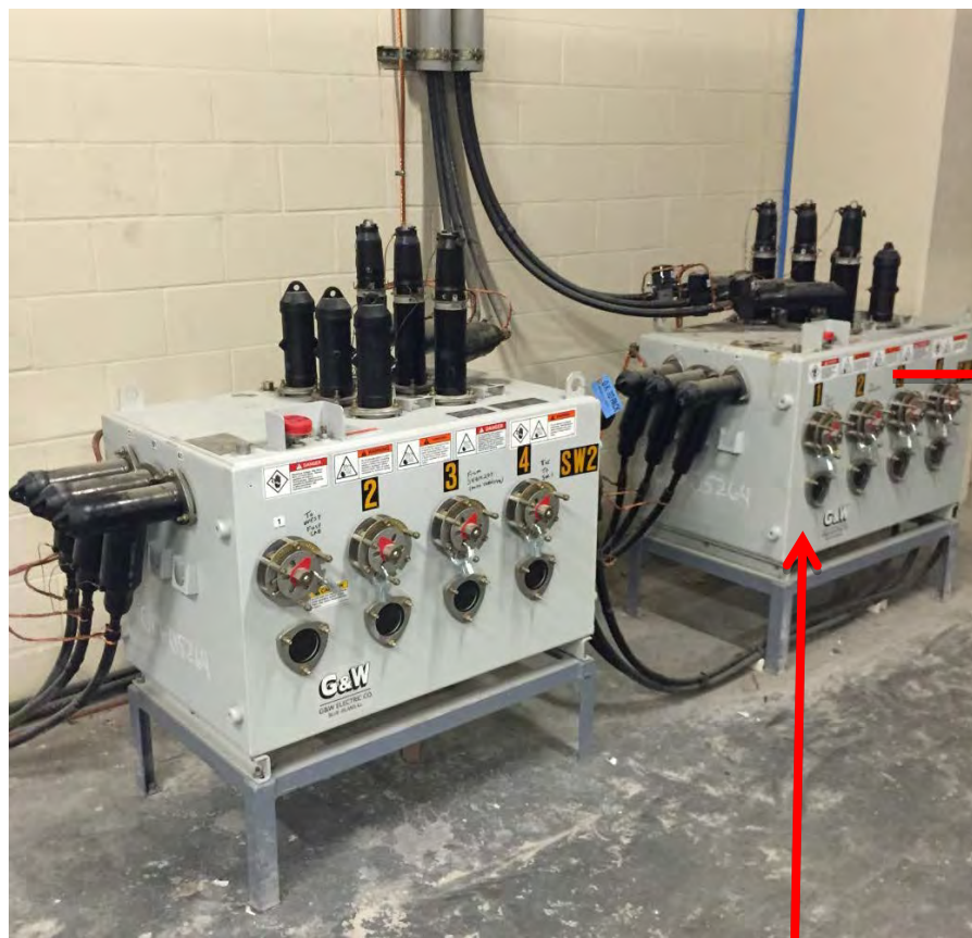
Fig. 2.1 Typical OUC Primary Switches
