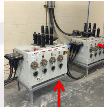
Typical OUC Primary Switches
