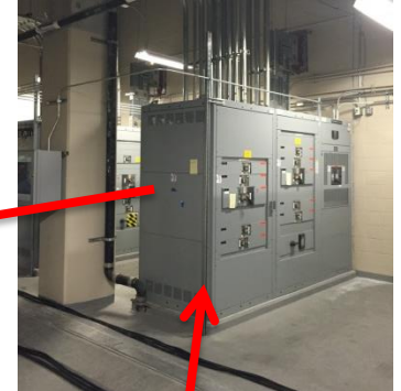
Typical 3000A Switchboard
