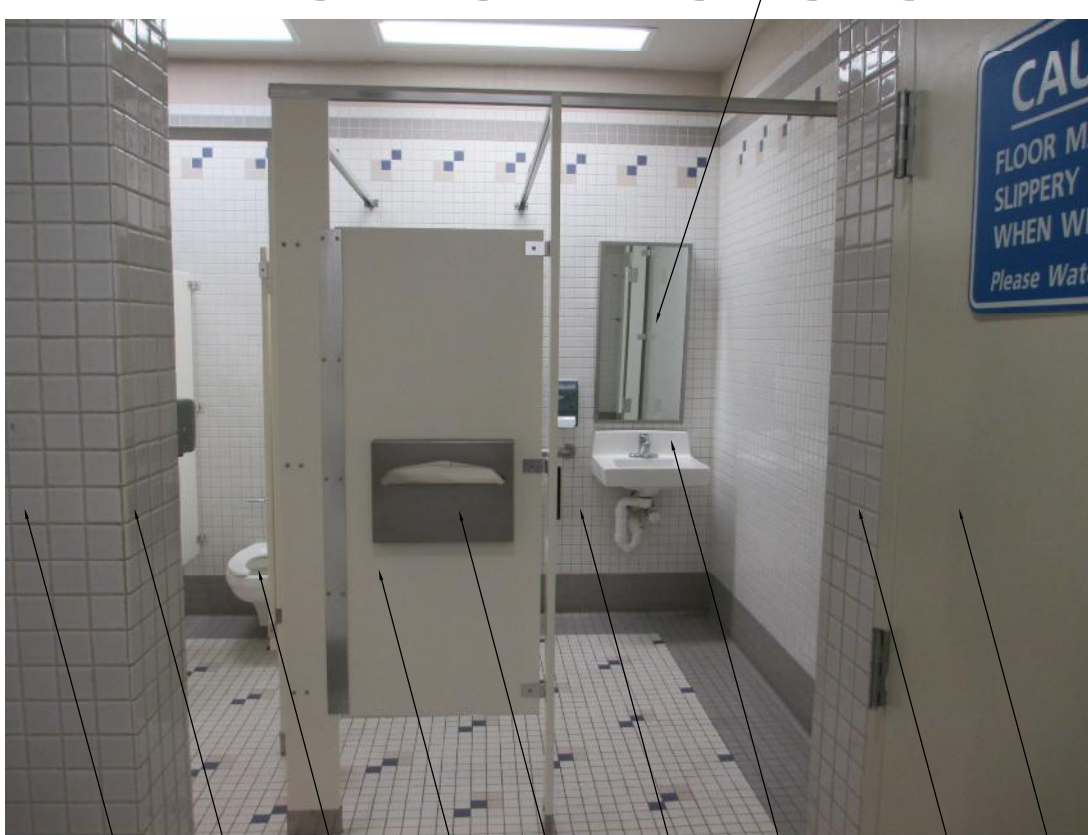
ADDITIVE NO. 01 CONCOURSE D - LEVEL 2 EXISTING IMAGES - ROOMS 263/264 scale: NTS E2 AD603
