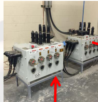
Typical OUC Primary Switches
