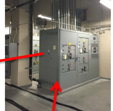
Typical 3000A Switchboard
