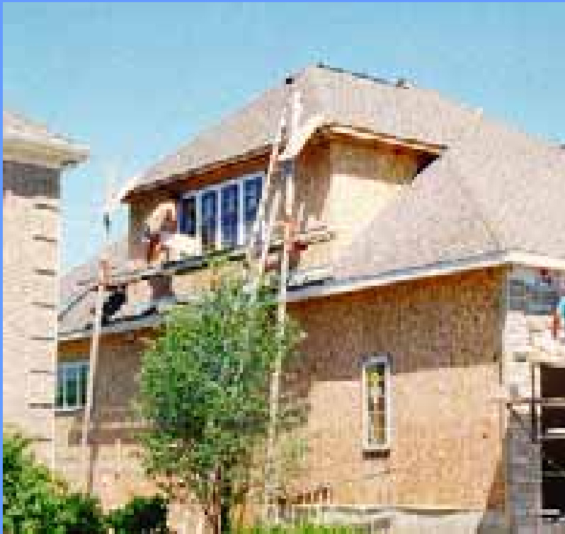
20' high -- No Guardrails
