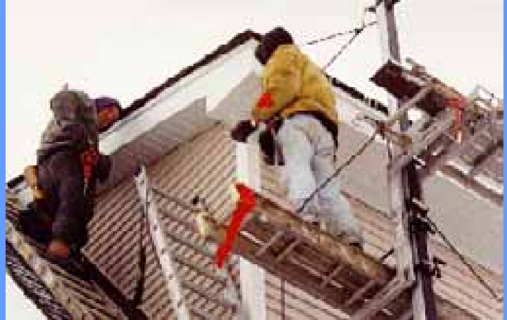
Chicken ladder used in lieu of fall arrest on roof.
